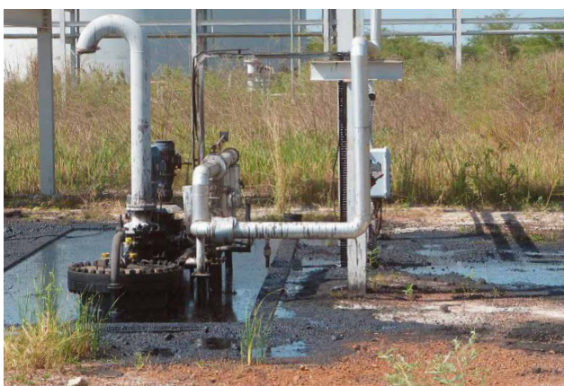
Oil leakages near Tharjath oilfield. Photo credit: Ministry of Petroleum
