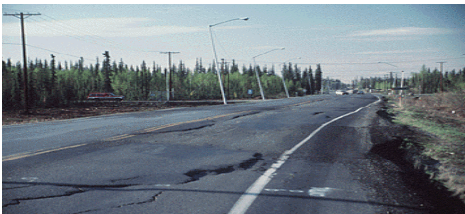
Figure 1. Photo of settlement and cracks on an Alaskan roadway due to warming of the permafrost foundation.
