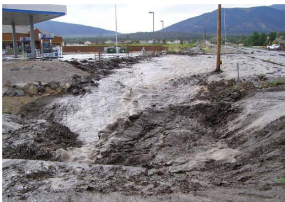
Flooding after the Schultz Fire overwhelmed established drainage infrastructure. Photo courtesy of Joanne Keene.
