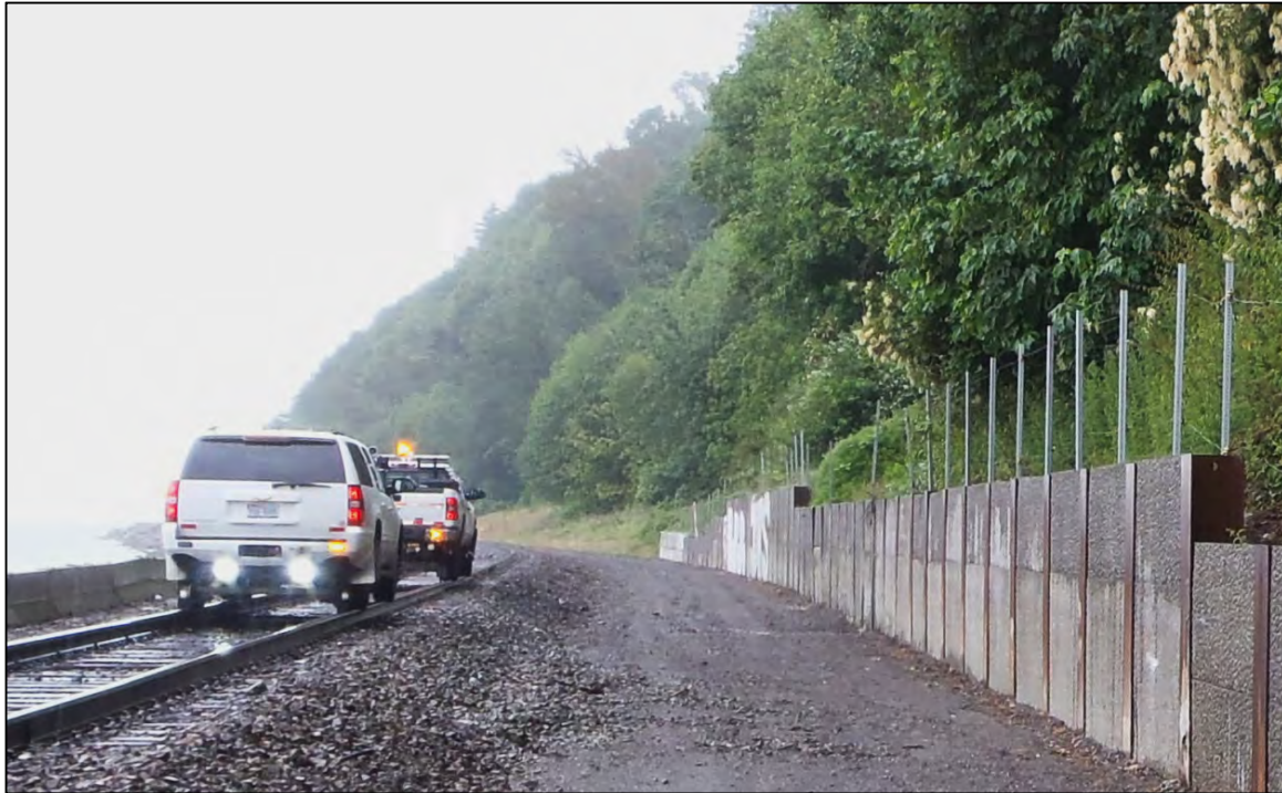
Figure 9. Slide fence on top of a wall along the BNSF right of way (photograph courtesy of BNSF).
