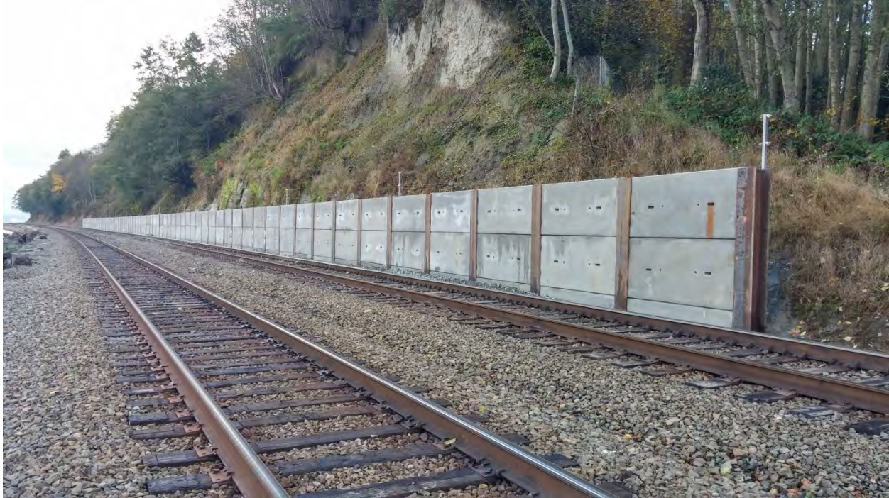
Figure 8. Debris containment wall along BNSF rail line consisting of steel “H” piles with precast concrete lagging to facilitate cleanout (photograph courtesy of BNSF).
