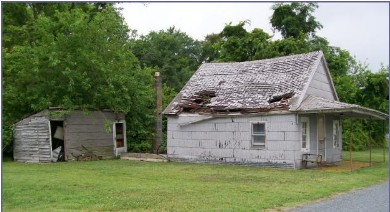
Property on Elliott Island Road in disrepair and likely little used.
