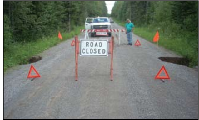
Damage to a forest road after the June 2012 rainstorm in northeastern Minnesota. Photo by Patrick Hampston, Superior National Forest.
