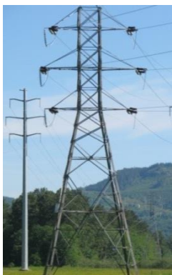
Transmission and Distribution
