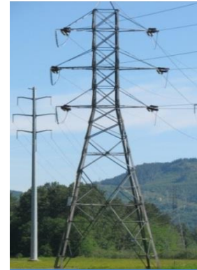
Transmission and Distribution
