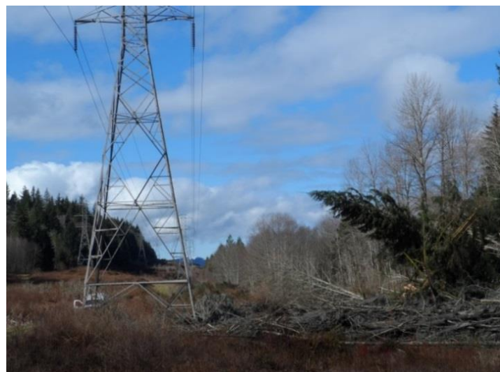
A steel tower of City Light's Skagit transmission line and debris deposited by the landslide near Oso, Wash. in March 2014. The debris caused minor damage to a tower.
