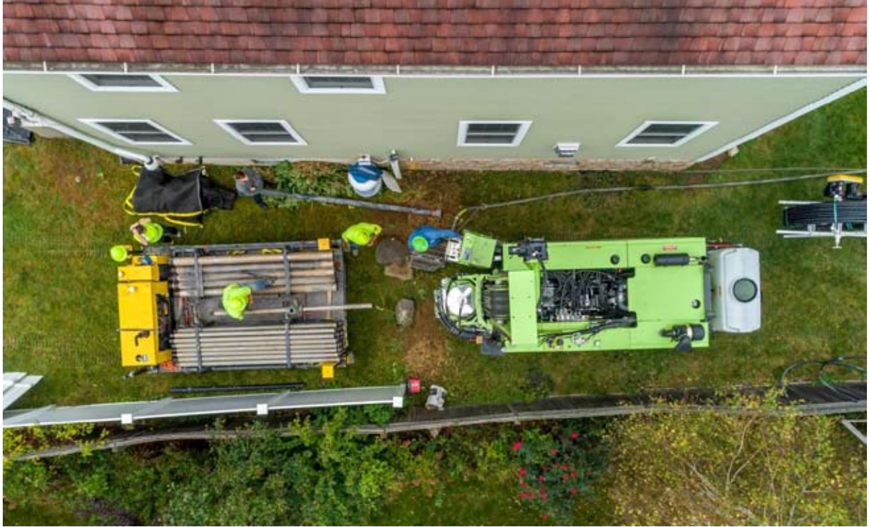
New York has used carbon auction funds to spur advancement of clean energy technologies, such as a faster and less expensive method of drilling and installing pipes in the ground for geothermal heating systems. Photo: Dandelion Energy
