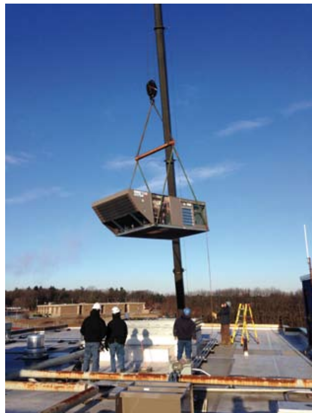
Through the Massachusetts Green Communities Program, carbon auction revenues helped pay for a more efficient heating and cooling unit at Chelmsford High School. Photo: Massachusetts Department of Energy Resources.
