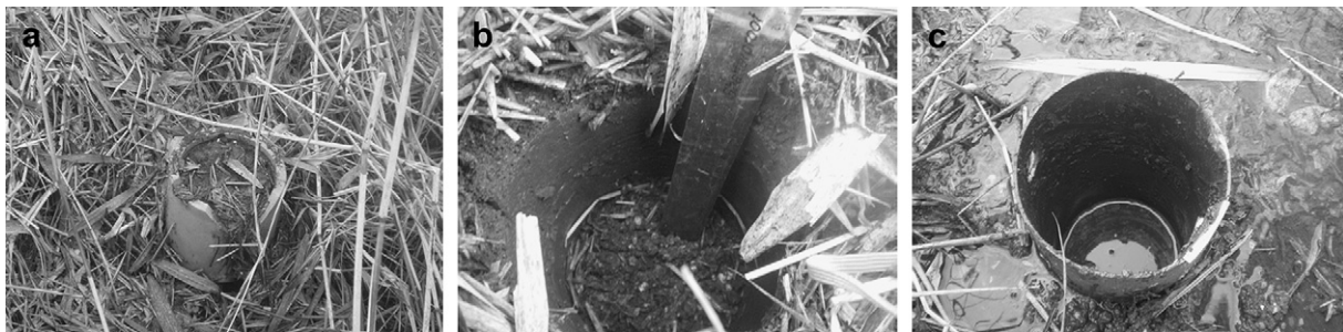
Fig. 2 – Photographs detailing the more prominent findings at the site, including a) Completely clogged inlet distributors, b) Surface sludge layers up to 200 mm thick at the inlet, c) two water levels at certain points in the system, representing disconnected overland and sub-surface flows.
