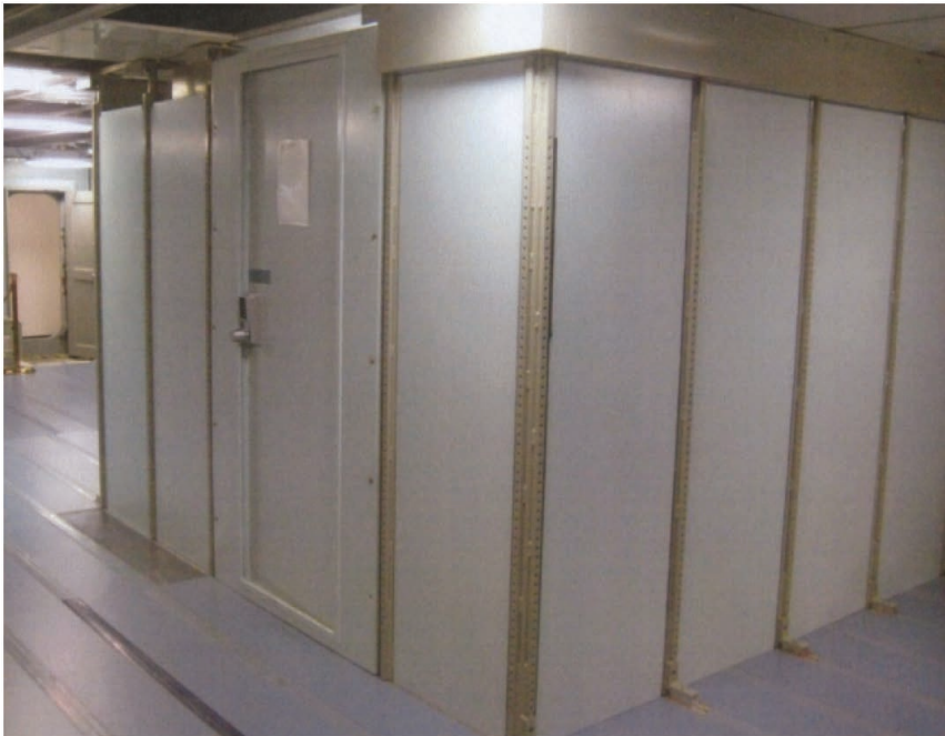
Figure C.4 Flexible Infrastructure Stanchions and Bulkheads
