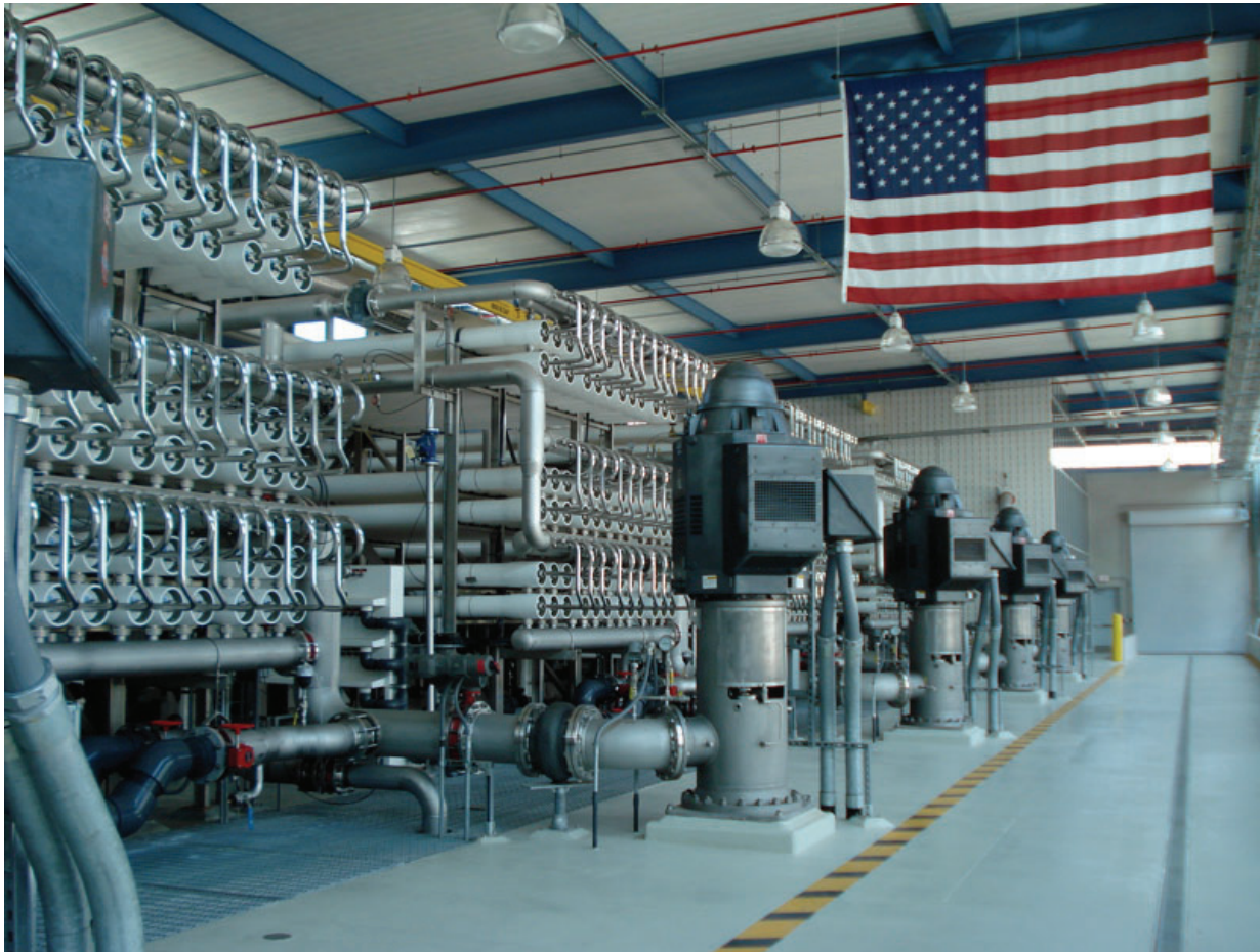
Figure 2.11. Kay Bailey Hutchison Desalination Plant
