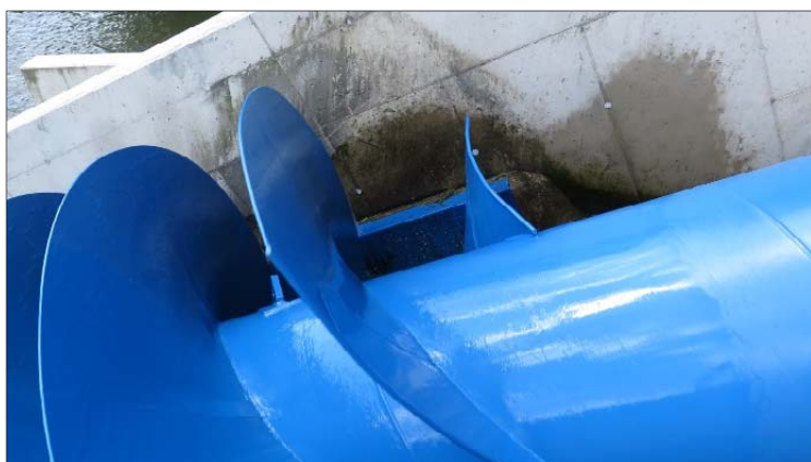
Figure 6.2. The upper part of the Archimedes screw turbine at Kuhlemühle in the Diemel. Photo by Eva B. Thorstad.
