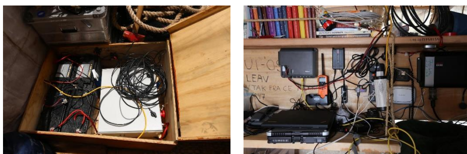
Figure 8 The 12V battery bank on Tupac, consisting of four 12V batteries is shown on the left; the white box is the inverter for the three-stage sampler and the most energy-demanding device on board. The rafts had a payload composed of electronic equipment for navigation and communication, shown on the right. The science/electronic desk on Tupac. On the table, a stack of PCs can be seen, including a
