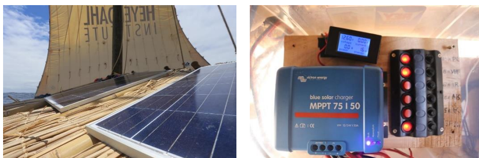
Figure 6 Solar panels were mounted on both rafts and provided the vessels with electrical energy. The solar charge controller, fuse panel and a voltmeter protected the electrical installation.
