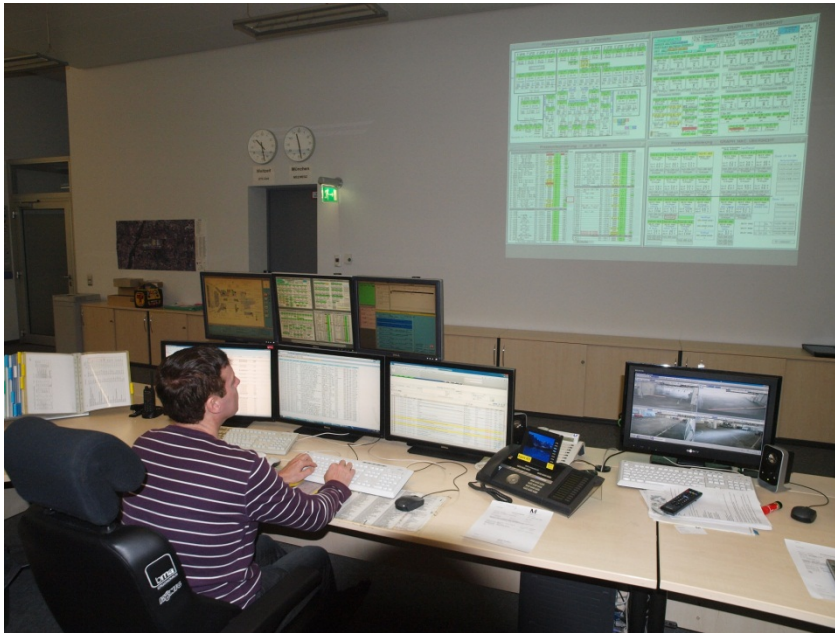
Figure 2.11 Workplace in the technical operations center with six monitors
