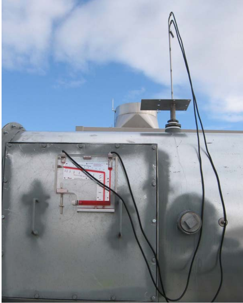
Figure 3.4. Slant Tube Manometer on 3430 Inspection Hatch Cover
