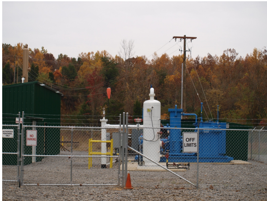
Figure 14. Gas collection and processing facility location.
