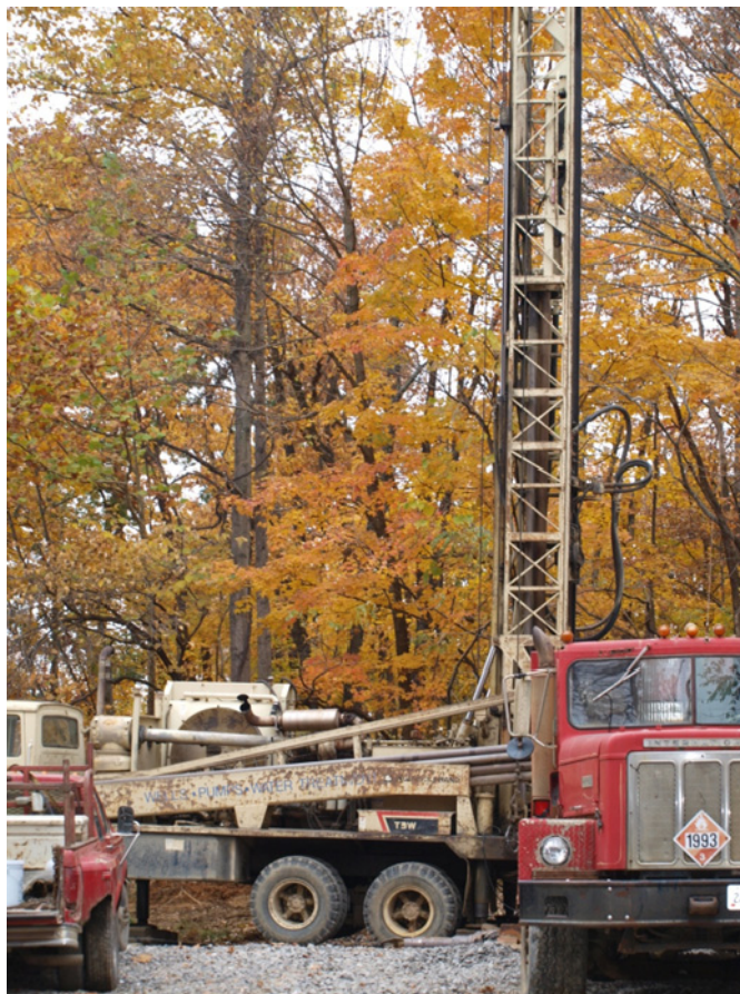
Figure 10. Drill pad design and rig used for drilling gas well down to the 600-700 ft. level.
