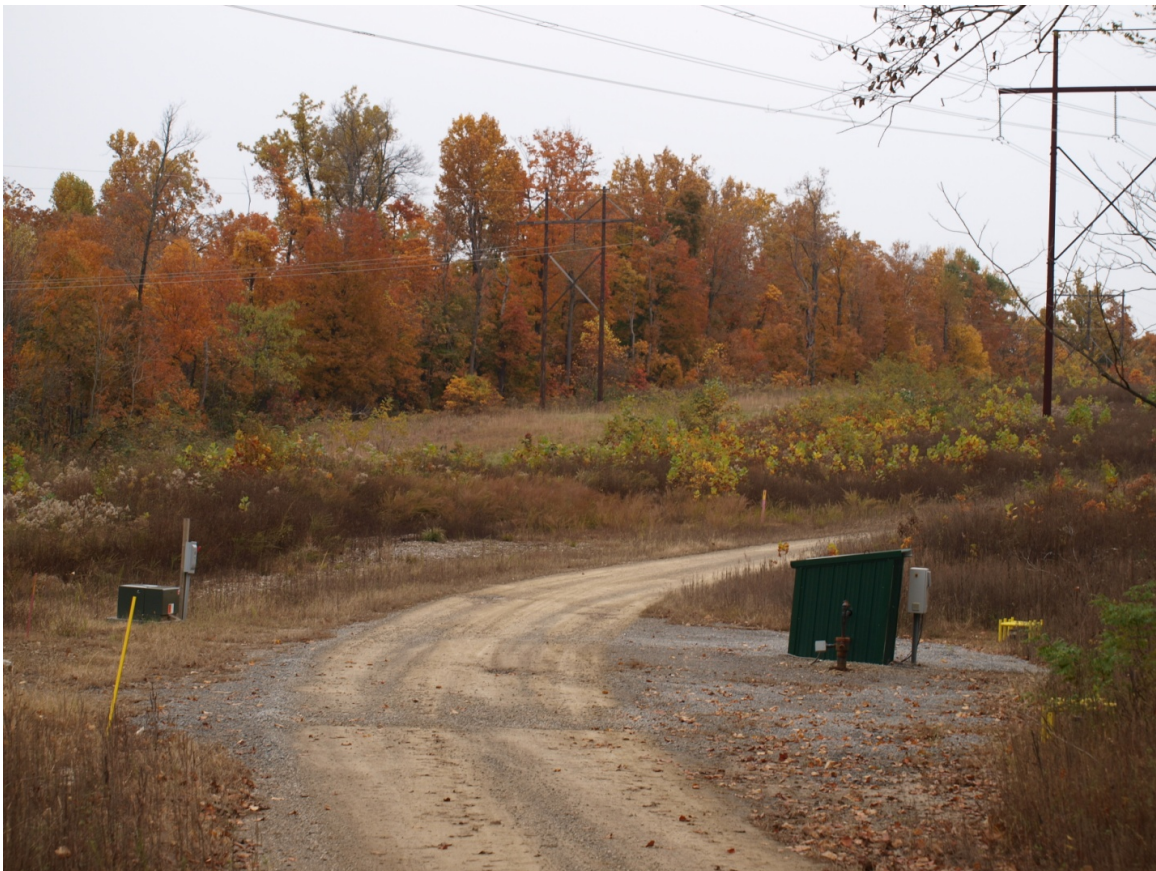
Figure 11. Complete gas well (yellow metal structure on the ground along right side), pump house, and electrical connection. Collection system buried along existing road.
