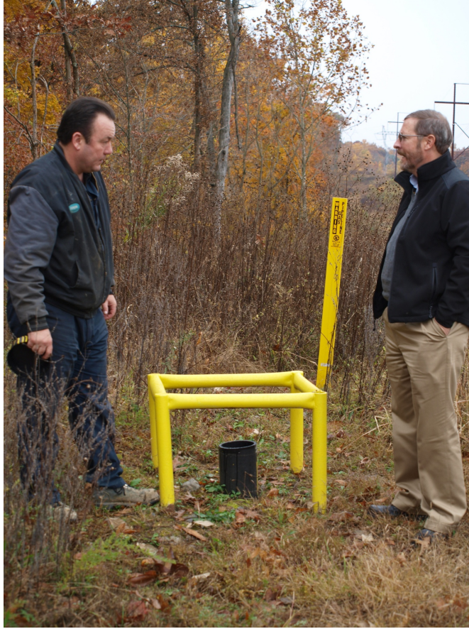
Figure 12. Frank Irvin, President of Trico (left), shows INL's Bob Breckenridge (right) how the gas collection wells are protected to ensure training operations at Ft. Knox do not impact the well heads.
