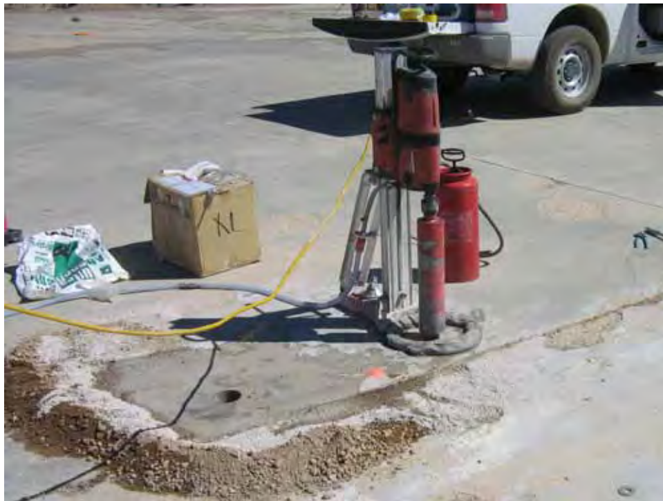
Photograph 49: Coring for Installation of Use Restriction Warning Signs around the Concrete Reactor Pad North of Building 3210, 09/01/2011
