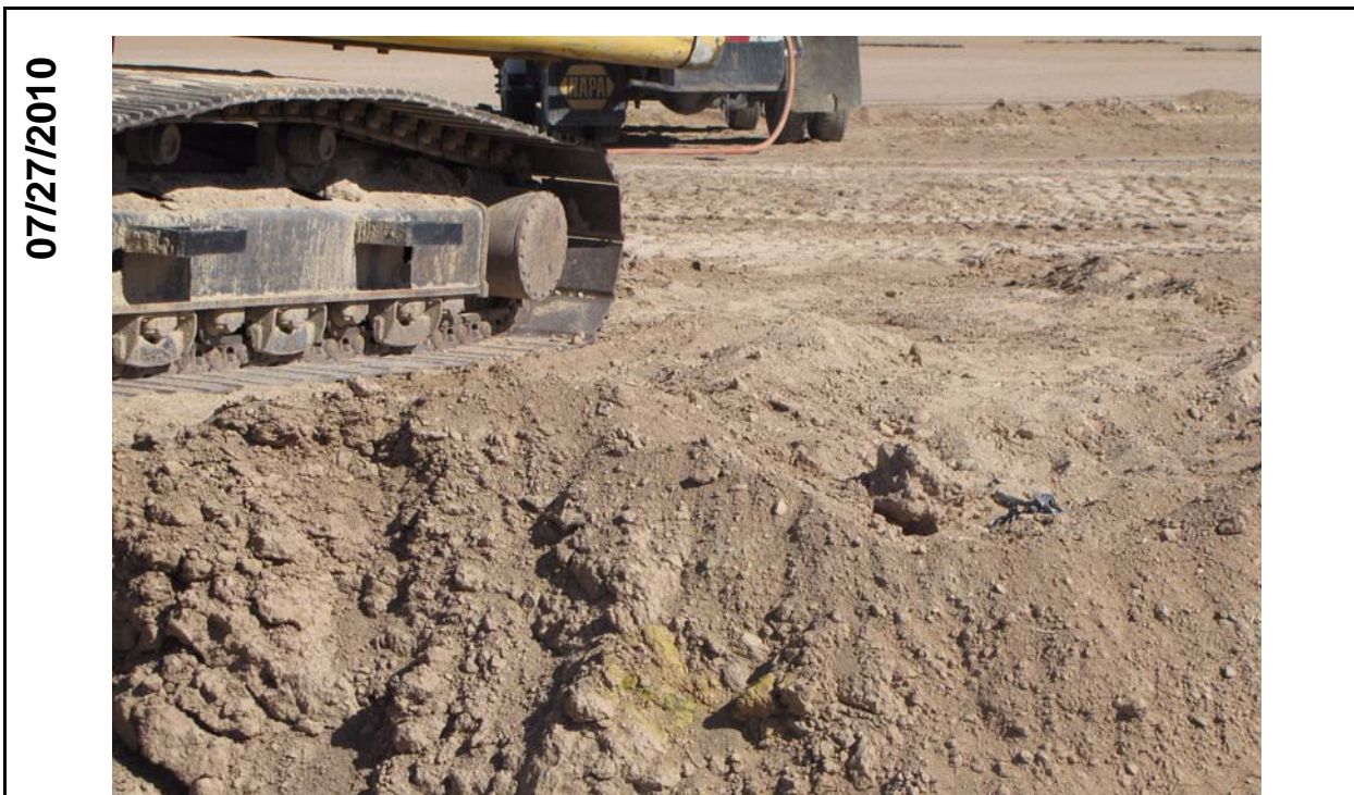
Figure 3-5 DU Soil Contamination in Excavation at CA-1 Site
