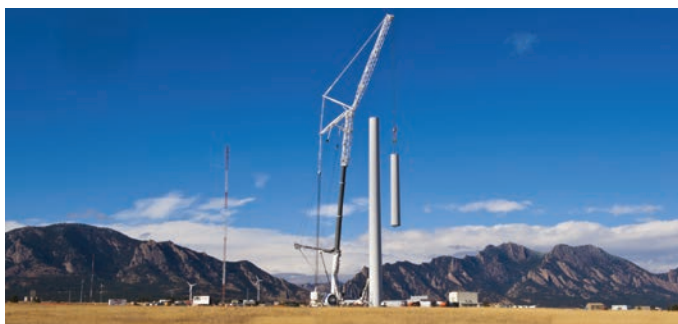
Installation of a 2.5 MW Alstom wind turbine at the NWTC. Photo by Dennis Schroeder, NREL/PIX 18888
