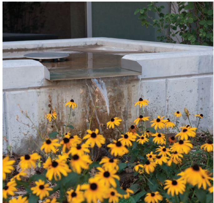
Rain water from the RSF passes through landscaped areas before release to the storm sewer. Photo by Robb Williamson, NREL/PIX 20954
