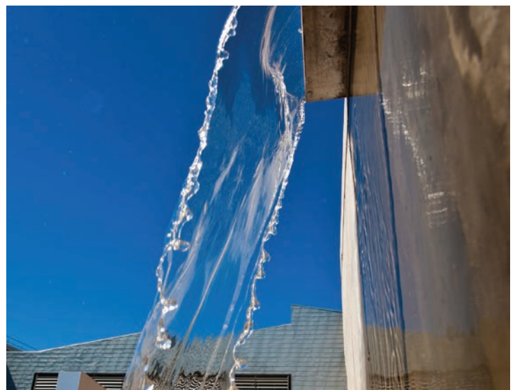
Melting snow from the roof of the RSF flows into containment structures and then into landscaping around the building. Photo by Dennis Schroeder, NREL/PIX 18640
