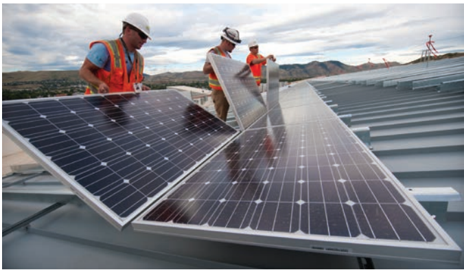
PV panel installation on the roof at the RSF. Photo by Dennis Schroeder, NREL/PIX 17843
