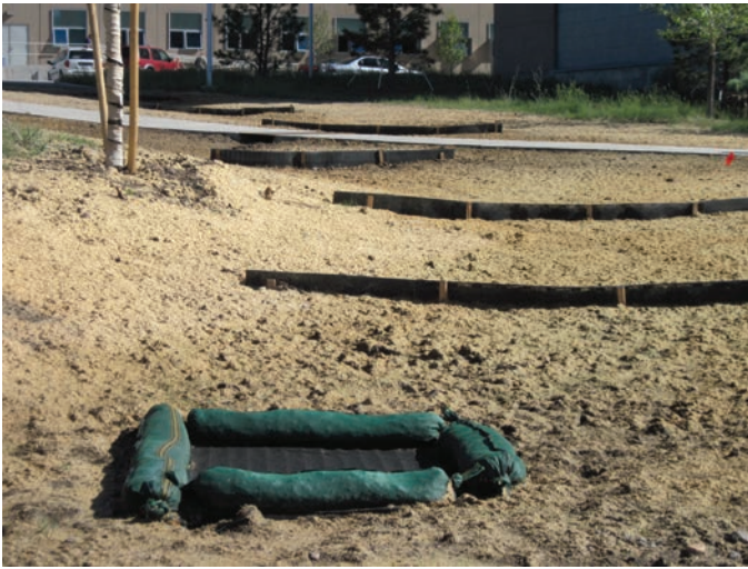
Layers of stormwater BMPs preventing erosion and controlling sediment. Photo by Kurt Schlomberg, NREL/PIX 21211
