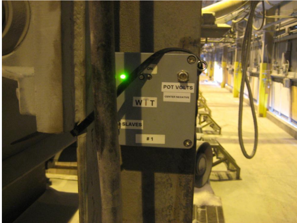
Fig. 9. Master mounted on the end of a pot at Alcoa’s Wenatchee plant.
