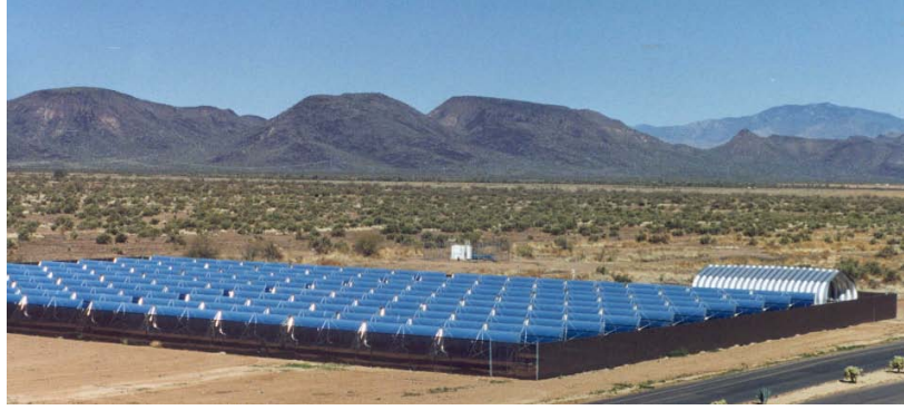
Figure 14. Solar industrial process heat system
