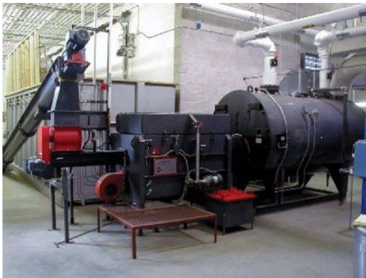
Figure 15. Biomass-fueled gasifier and boiler
