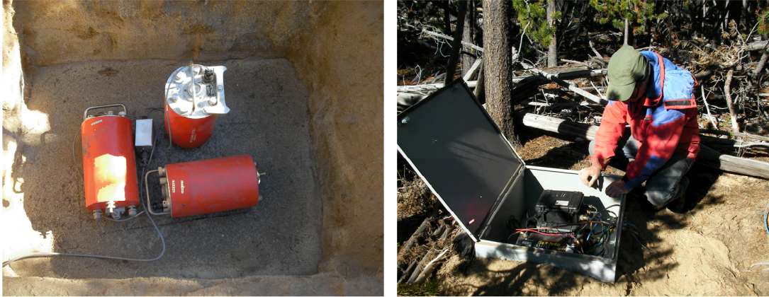
Site installation: Left: seismometers and resistor box on concrete pad. Right: digitizer, batteries, and all cables are well protected in the Hoffman box.
