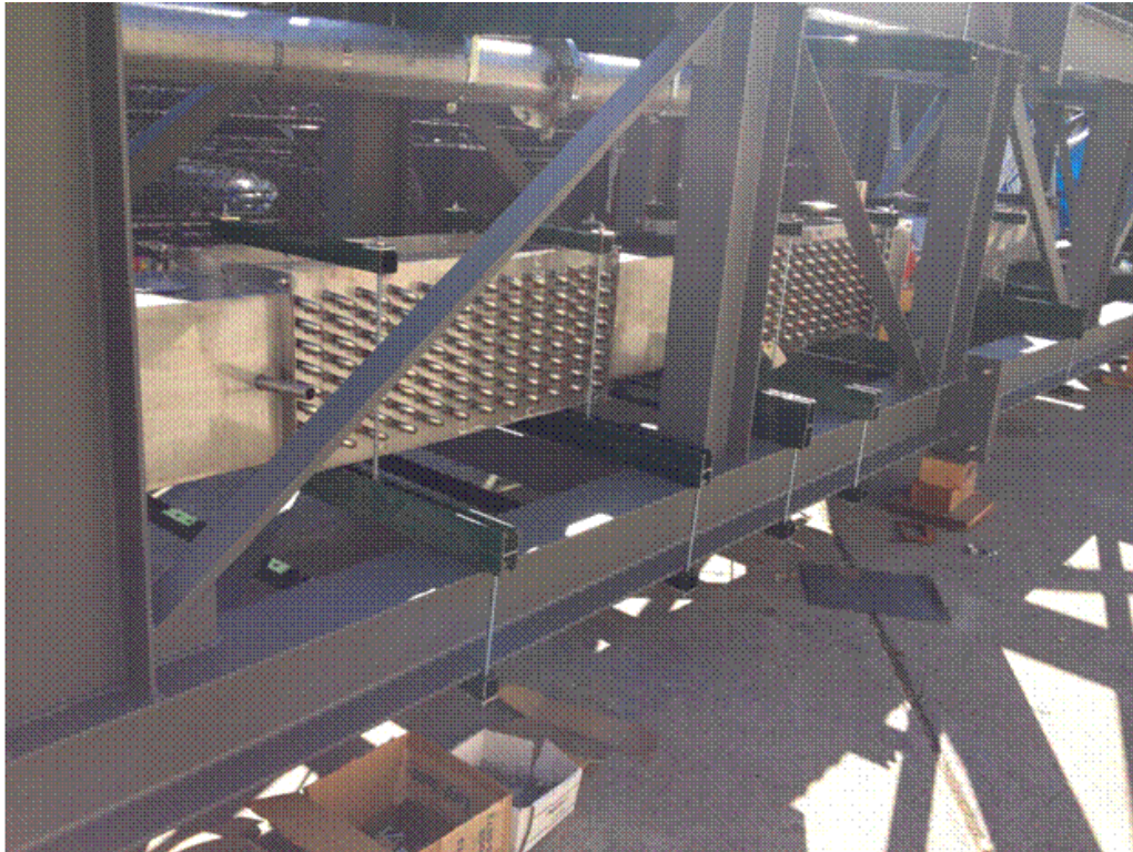
Figure VI-15. Photograph of a heat exchanger for recovering thermal energy from the sorbent granules.
