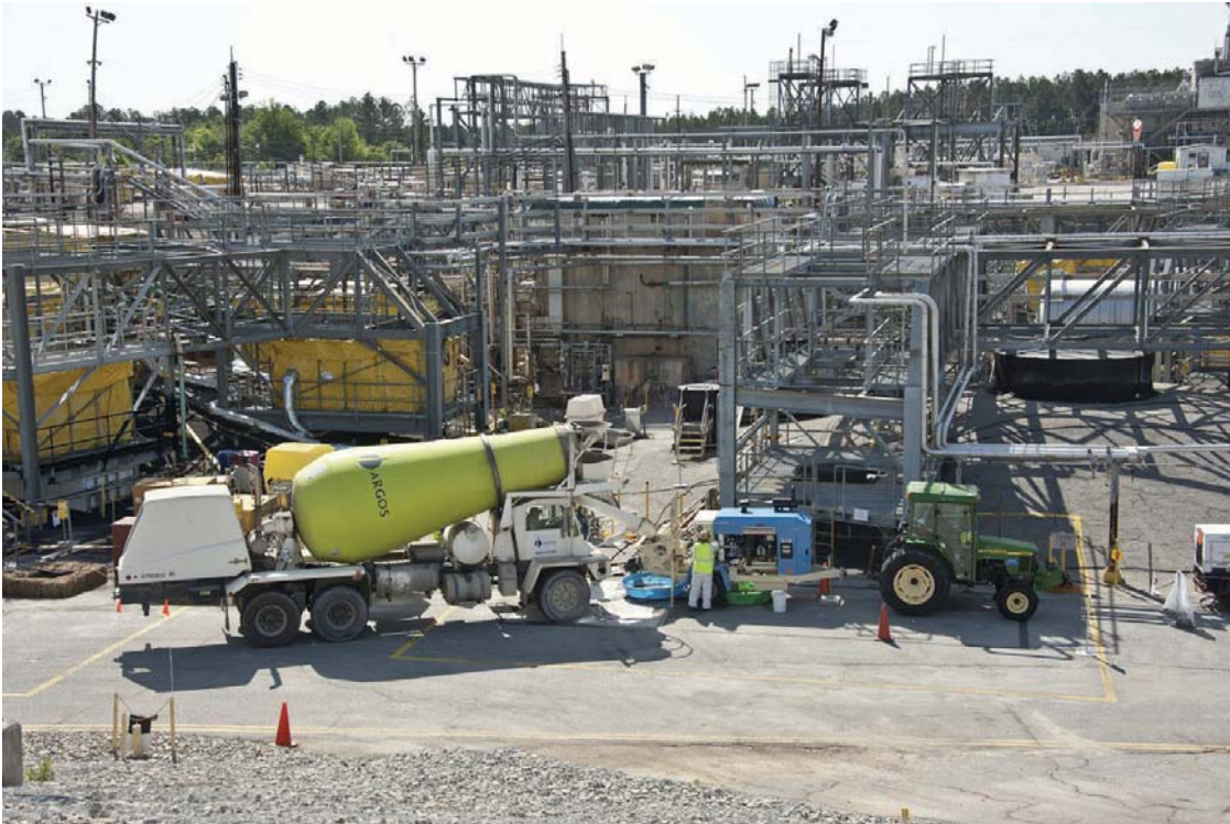
Figure 3-1 SRS Workers Pump Grout from a Concrete Mix Truck to Tank 18F.
