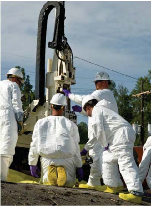
Figure 2-7 Mercury Characterization using Traditional Soil Sampling Techniques
