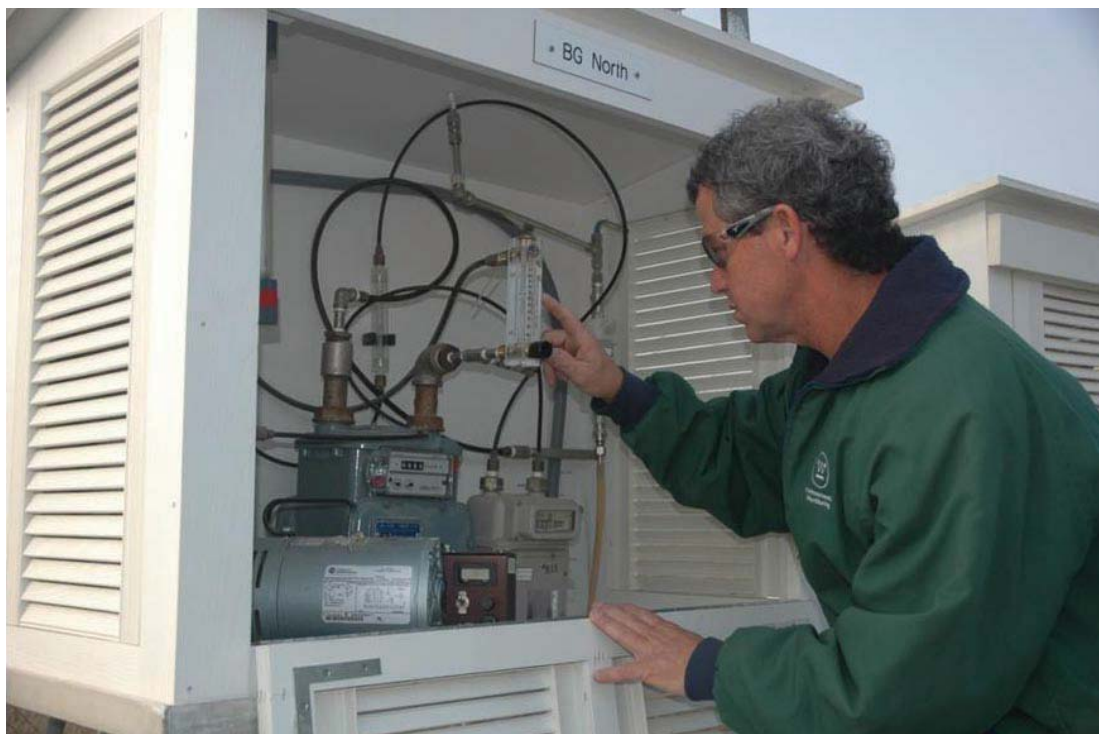
Figure 5-2 Environmental Monitoring Field Technician Reads Air Flow at the Burial Ground North Air Surveillance Station
