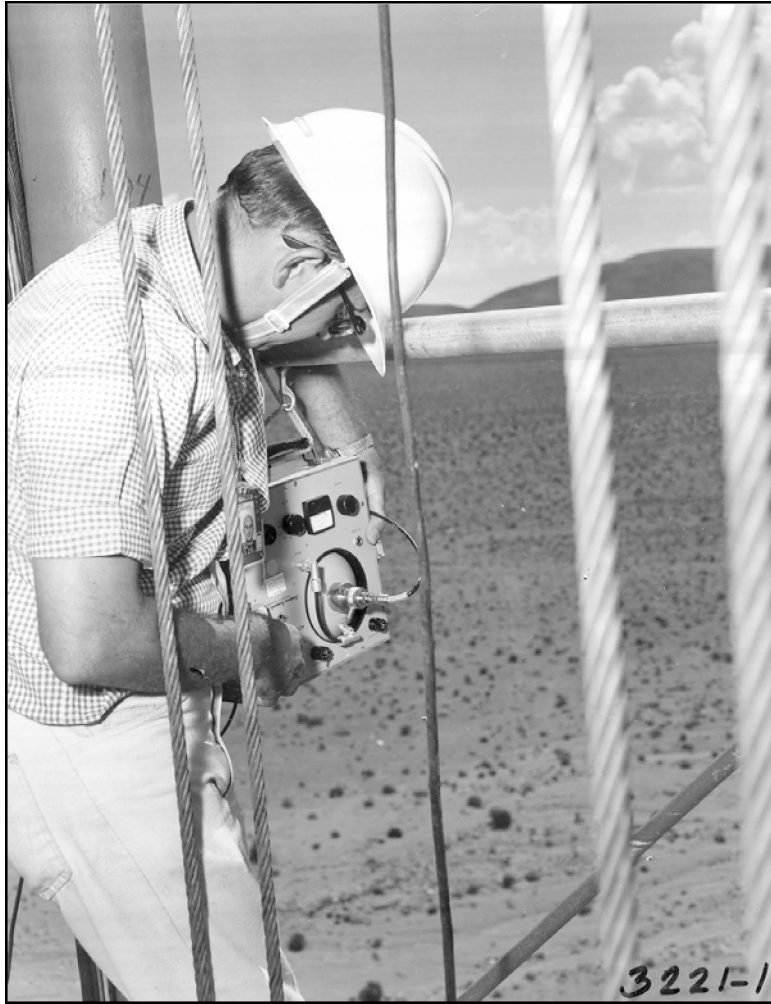
Photo 85. Technician rigging BREN Tower with instrumentation for the sonic boom tests. Photo taken August 26, 1970 (Photo 3221-16 on file at NNSA/NSO Nuclear Testing Archive).
