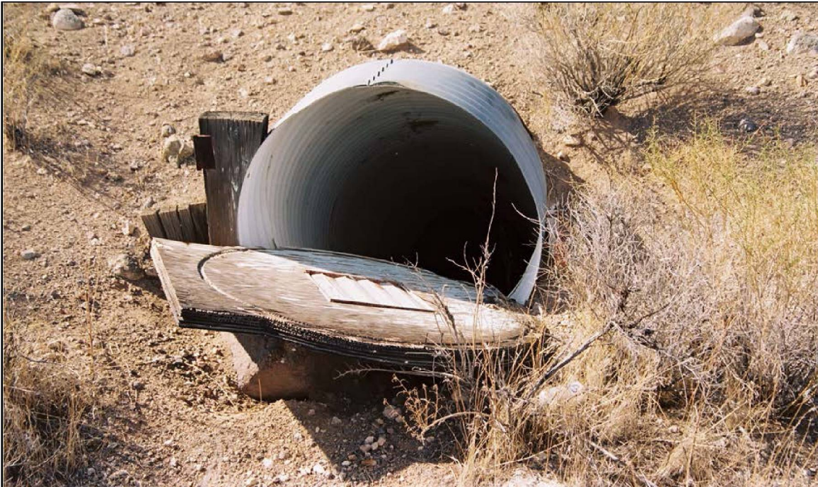
Photo 22. Detail of entrance to the underground civil defense shelter. Wooden door has fallen open since the June 2004 field inspection. View down and to the west. Photo taken by DRI on November 1, 2006 (on file at NNSA/NSO Curation Facility).
