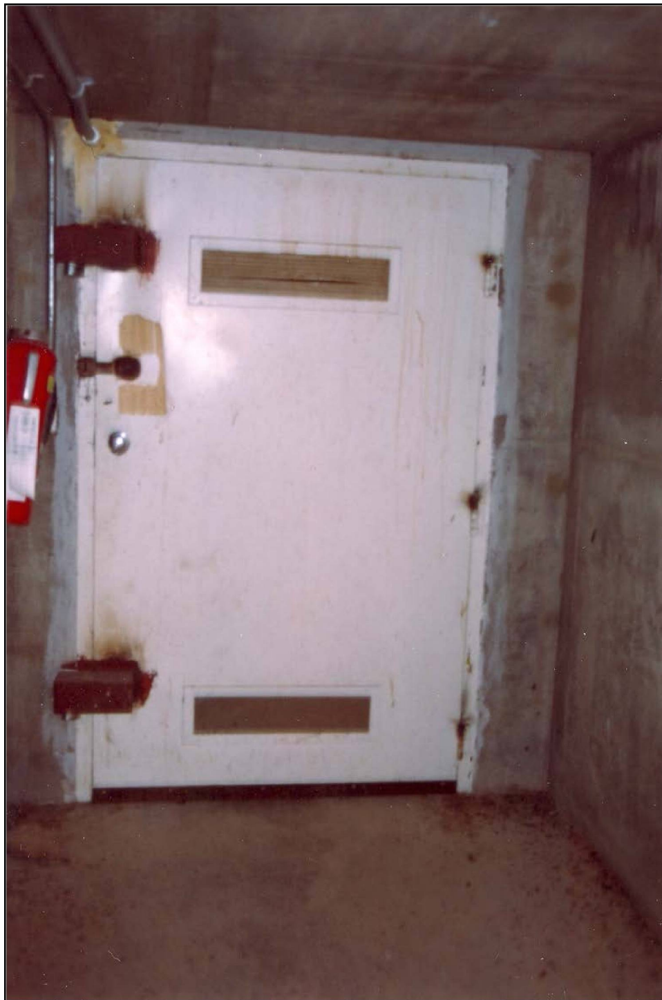
Photo 14. Entry door leading to the interior of the Control Bunker. View is from the tunnel facing west. Photo taken by DRI in June 2004 (on file at NNSA/NSO Curation Facility).
