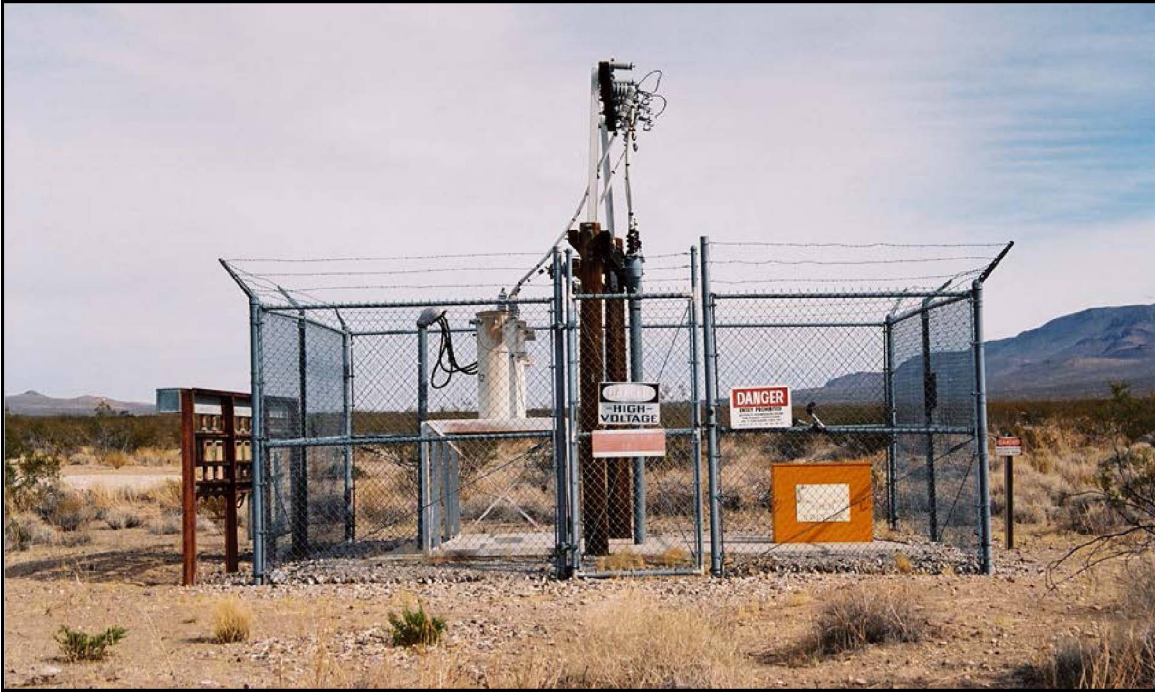
Photo 82. Substation 28-2 which serviced the remote support trailer park and heliport for Operation HENRE. The edge of the graded area for the trailer park is at the left edge of the photo. The heliport was about 250 ft south of the substation. View is to the east. Photo taken by DRI on November 1, 2006 (on file at NNSA/NSO Curation Facility).
