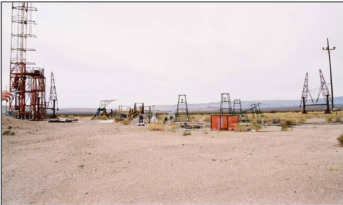
Photo 10. View of the Control Bunker, Substation 28-1, and some discarded equipment. Photo taken from BREN Tower's 31-ft high main work platform, November 1, 2006. View is to the east-southeast (on file at NNSA/NSO Curation Facility).
