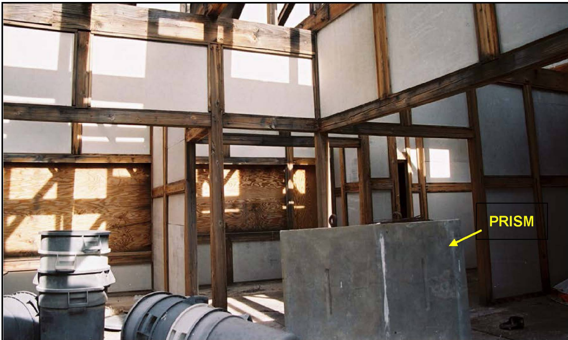
Photo 46. The concrete prism remains in place inside the analog Japanese House. View is to the north-northeast. Photo taken by DRI on November 1, 2006 (on file at NNSA/NSO Curation Facility).
