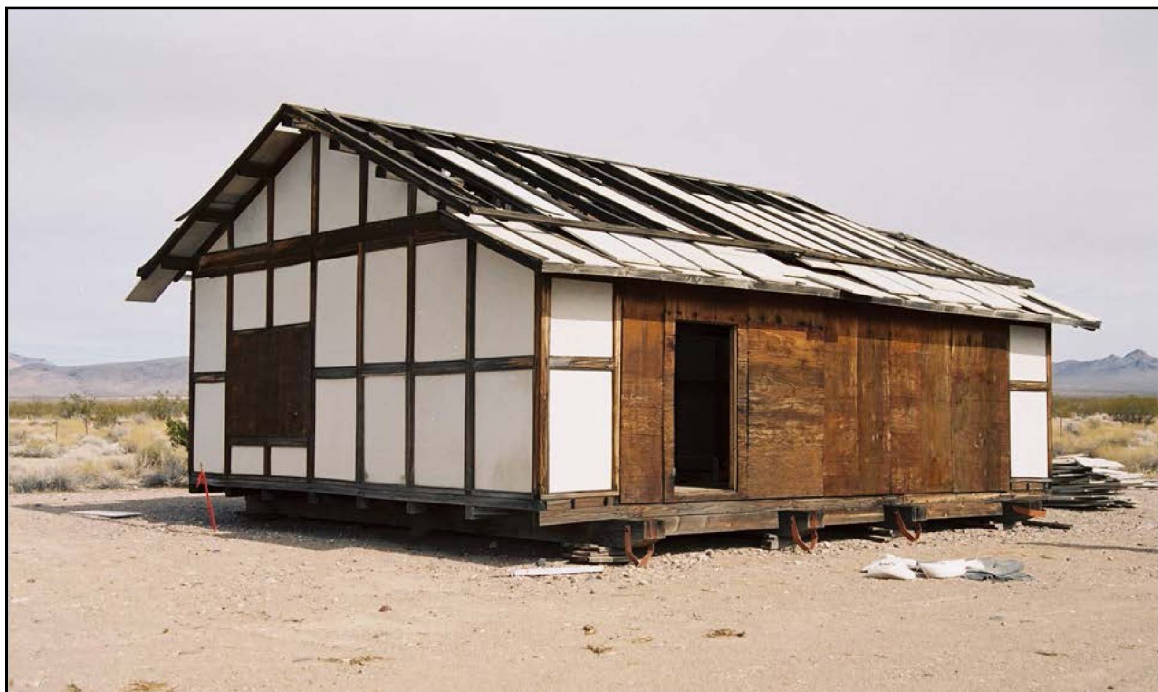
Photo 42. West and south elevations of the analog Japanese House in November 2006. View is to the northeast (on file at NNSA/NSO Curation Facility).
