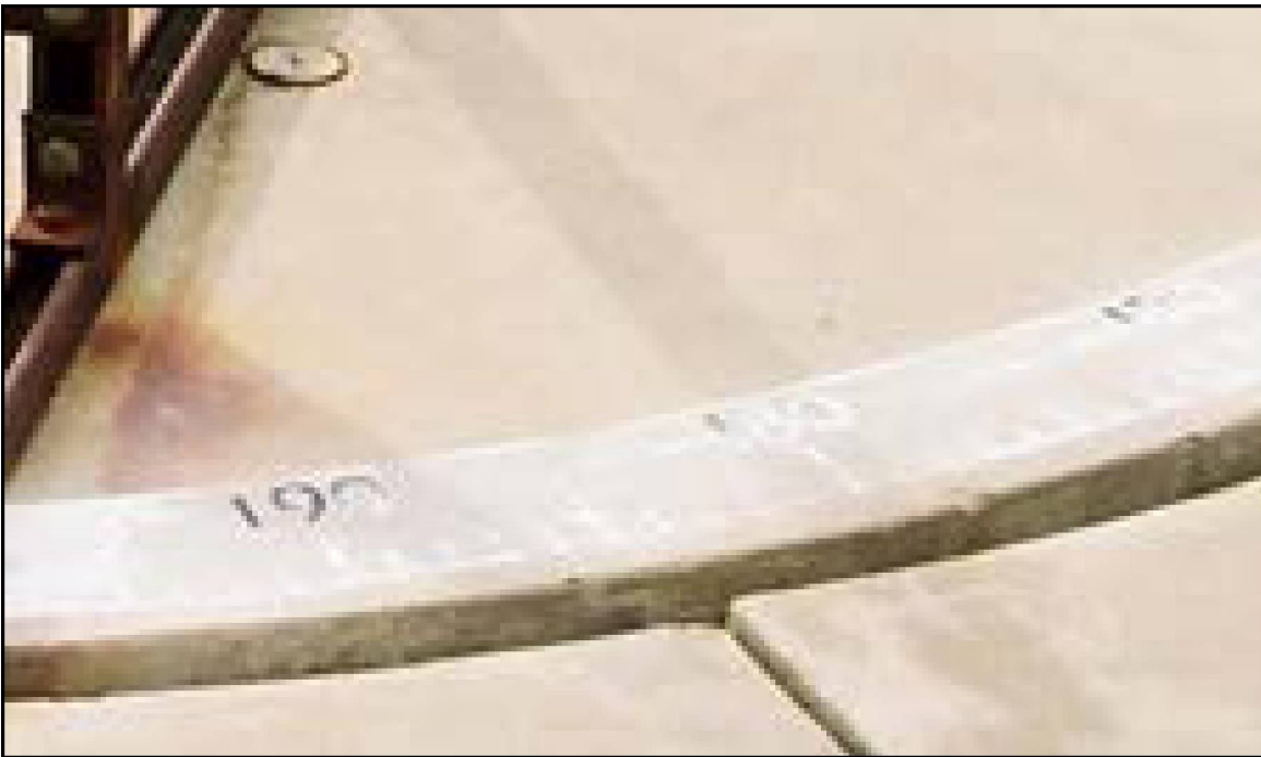
Photo 73. Detail of the Program 9 turntable and the degree markings painted on the rotating platform. Photo taken by DRI on November 1, 2006 (on file at NNSA/NSO Curation Facility).
