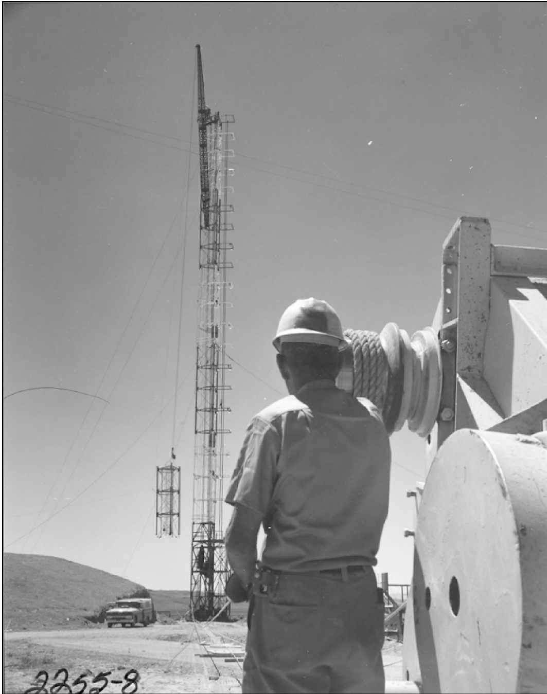
Photo 2. BREN Tower being reassembled at NTS Area 25, May 12, 1966. Temporary guy wires stabilize the tower during construction. The earth mound covering the Control Bunker appears on the left behind the truck. View is to the west (Photo 2255-8 on file at NNSA/NSO Nuclear Testing Archive).
