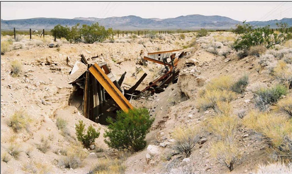
Photo 77. The covered trailer revetment located 750 ft from the base of BREN Tower was used to shelter the recording trailers for Operation HENRE experimental Programs 2 and 9. The wood and metal cover has collapsed. View is to the northeast. Photo taken by DRI on November 01, 2006 (on file at NNSA/NSO Curation Facility).
