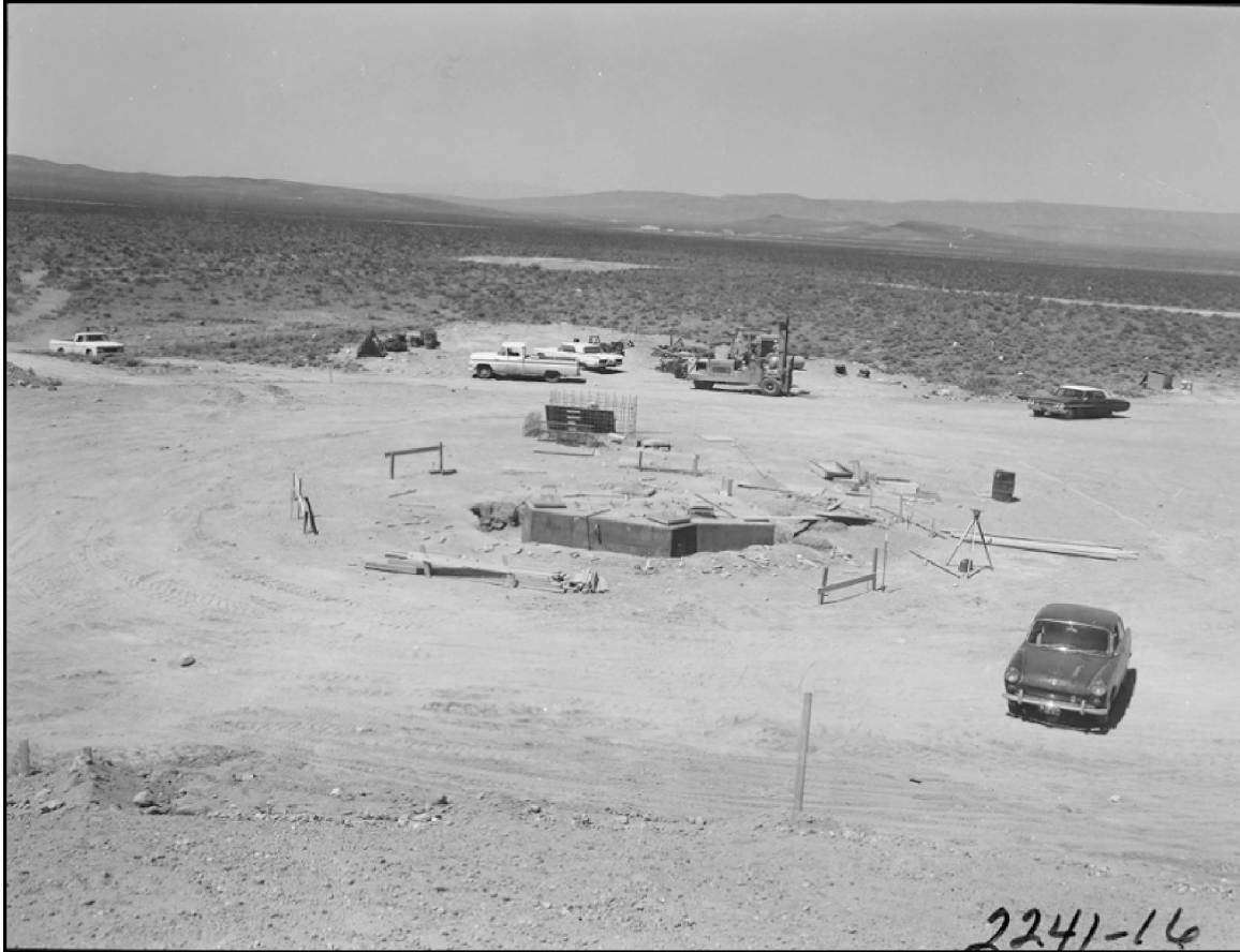
Photo 1. The newly completed foundation for BREN Tower's new location in NTS Area 25. Photo taken May 2, 1966. View is to the northwest (Photo 2241-16 on file at NNSA/NSO Nuclear Testing Archive).
