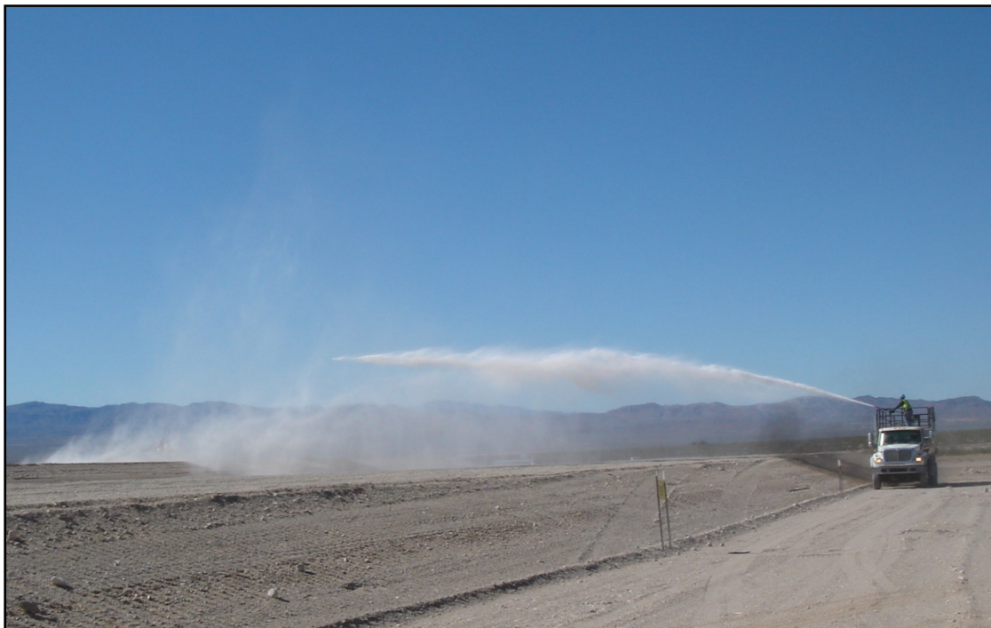
Figure 7-3. Application of Soiltac ® on the 92-Acre Site following deep ripping in April 2011 (Photo by D. Anderson, April 28, 2011)
