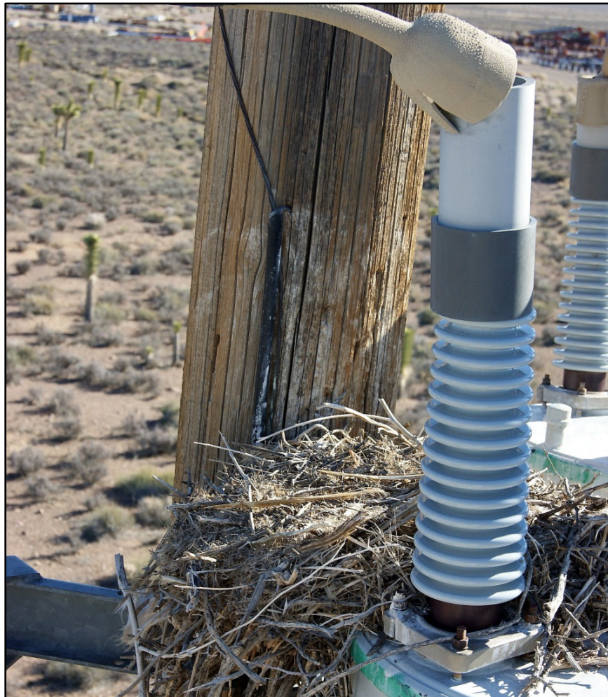
Figure 6-25. Photo of red-tailed hawk nest in Area 1 retrofitted with insulation bushings (top) on electrified lines to reduce electrocution risk
