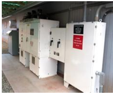
Figure 5. String inverter. Photo by Warren Gretz, NREL 07985
