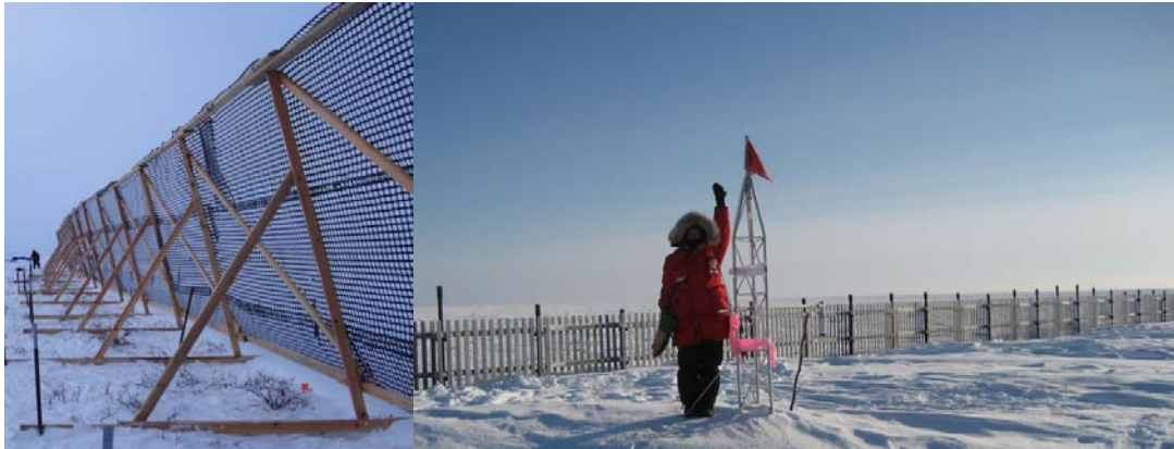
Figure 3. Photograph on the left shows Wyoming-type snow fence near Franklin Bluffs, North Slope of Alaska (September 2010). The photograph on the right shows a 4 m tall pole-supported snow fence in Barrow half hidden under the snowdrift (March 6, 2008). The researcher is standing on top of the snowdrift next to a 5 m tall instrumentation tower almost buried under the snow.
