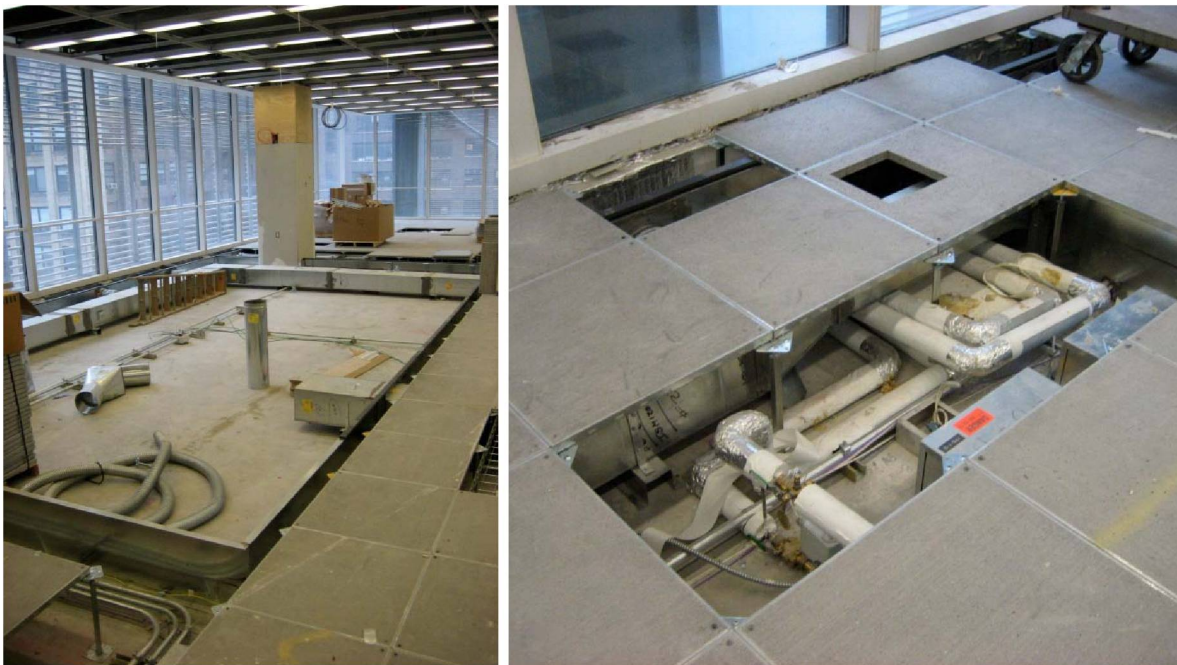
Figure 18. Images of the initial construction of the underfloor air distribution system. Copyright: LBNL.
