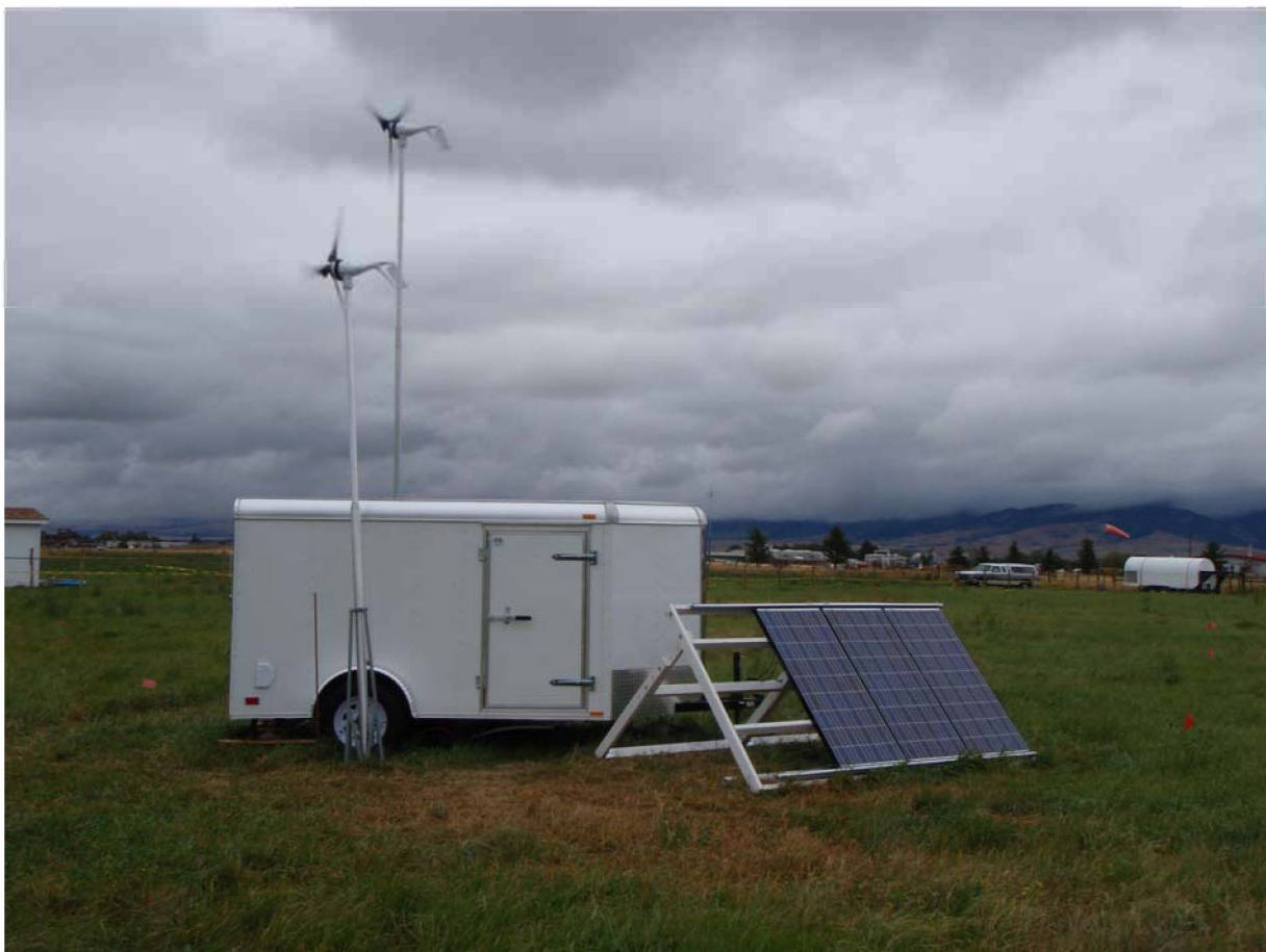
Figure 4.1. Power Supply System: Wind Turbines, Turbine Towers, Solar Array, and Trailer as Deployed at ZERT Site in 2008
