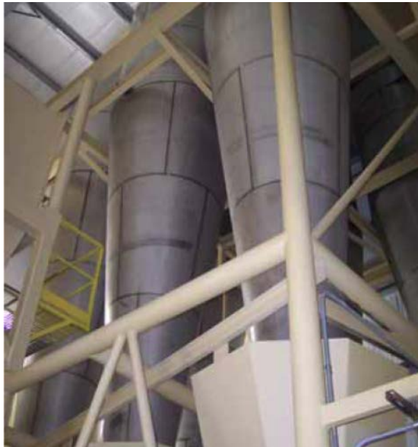
Figure 22. Cyclones for separating out water vapor
