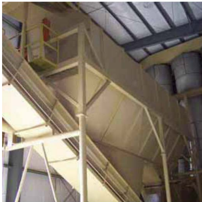
Figure 16. Biomass in-feed system
