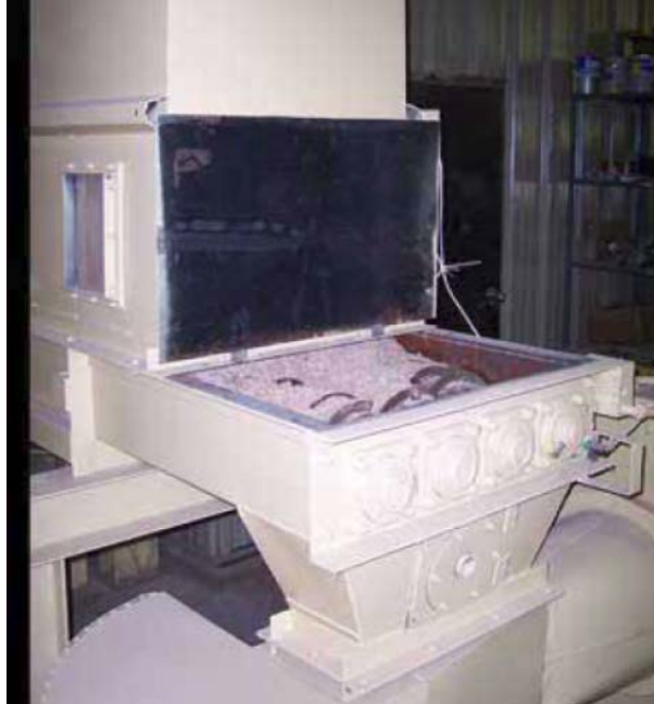
Figure 21. Burner feed augers and metering bin
