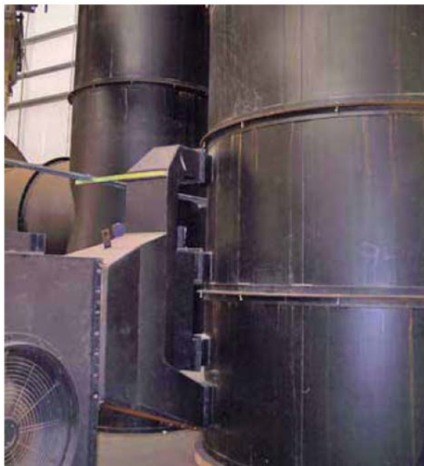
Figure 20. Biomass boiler for dryer
