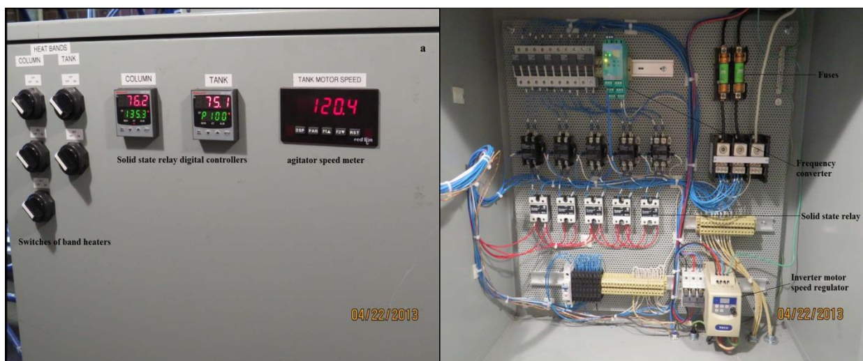
Figure 4B-3. Photographs of the electrical control panel.
