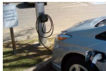
Figure 6-7. EVSE Level 2 charging station.
