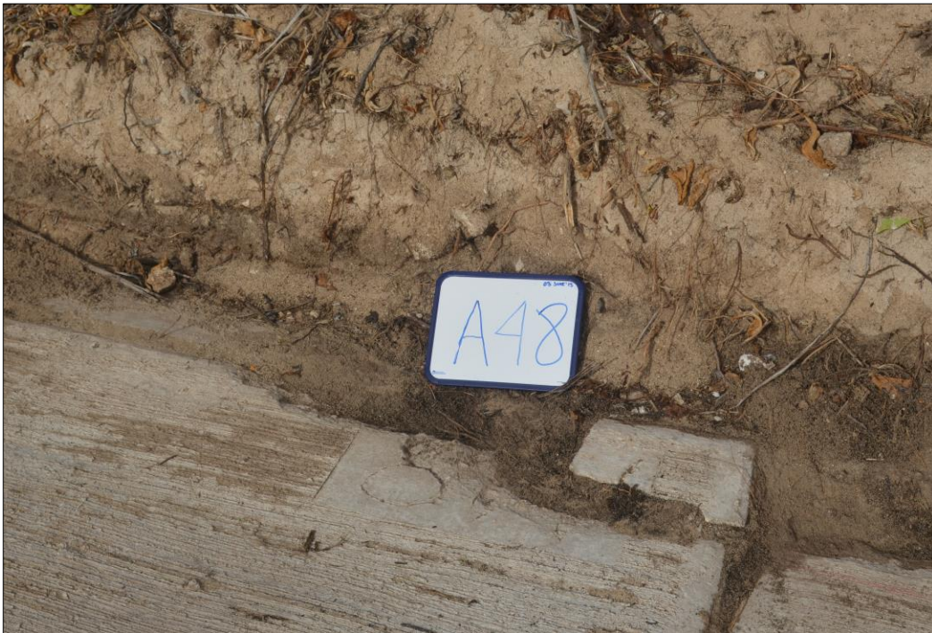
Fig. 29. Spalling and cracked concrete along the seam adjacent to the keywall in the left-hand corner of panel A48.
