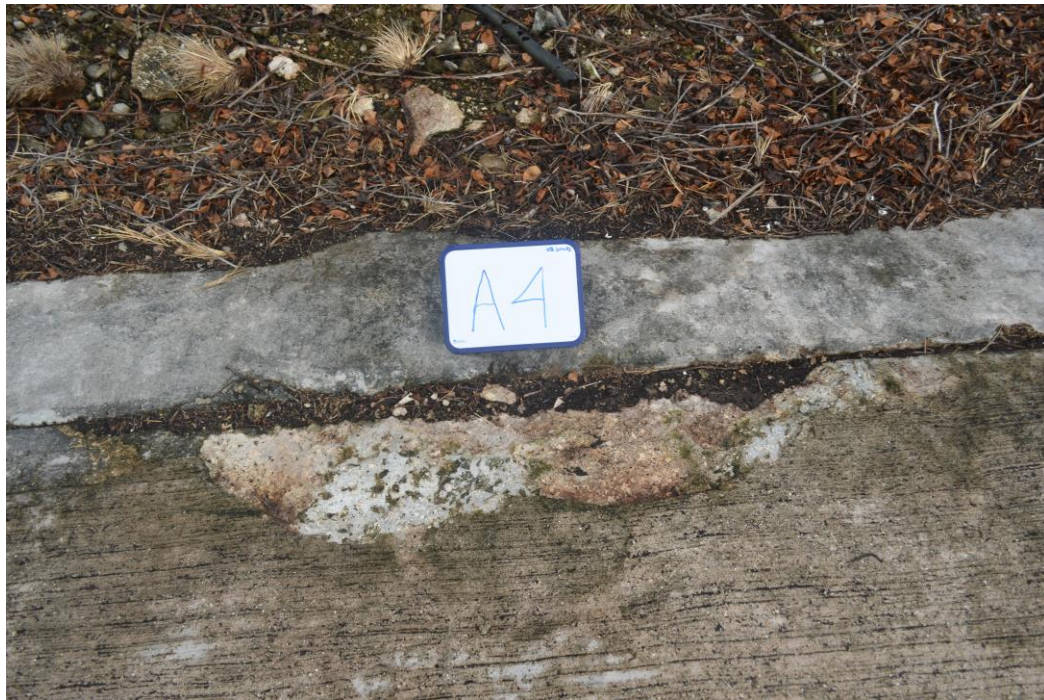
Fig. 19. Spalling of concrete along the bottom seam adjoining the keywall on panel A4.
