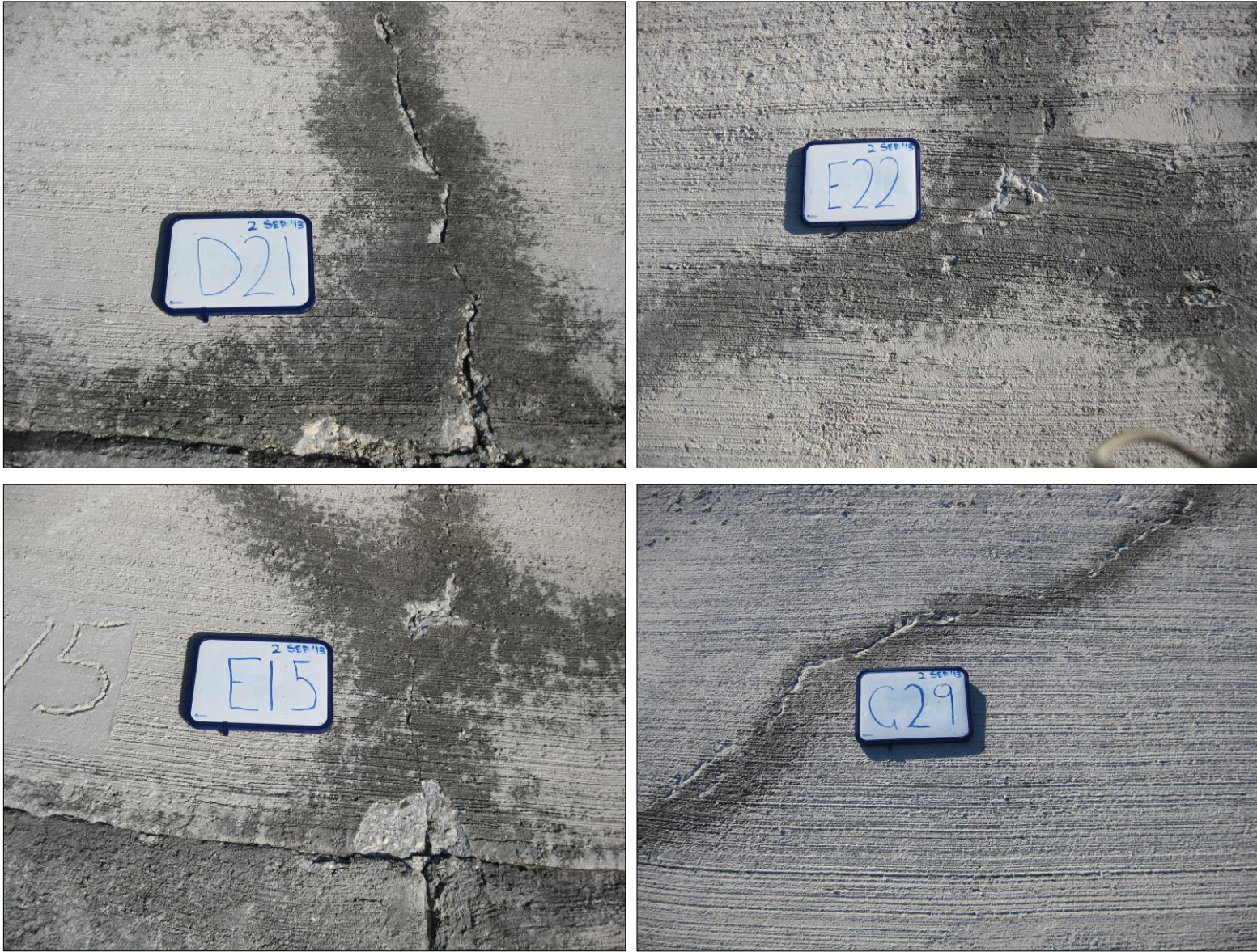
Fig. 38. Visually-defective concrete panels (D21, E15, E22, G29) showing minor to moderate size cracks with chipped “spalled” edges.
