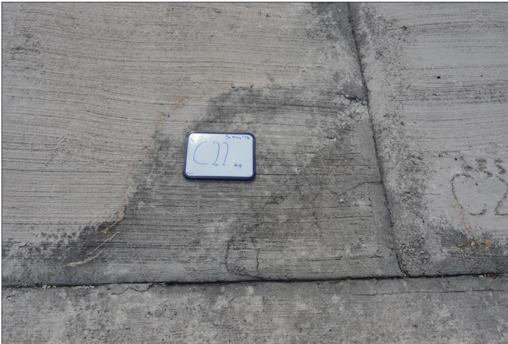
Fig. 35. Cracked concrete with spalled edges on the bottom, right-hand corner of panel C22_duplicate (position C24) [Refer Appendix I for extra panel positioning].
