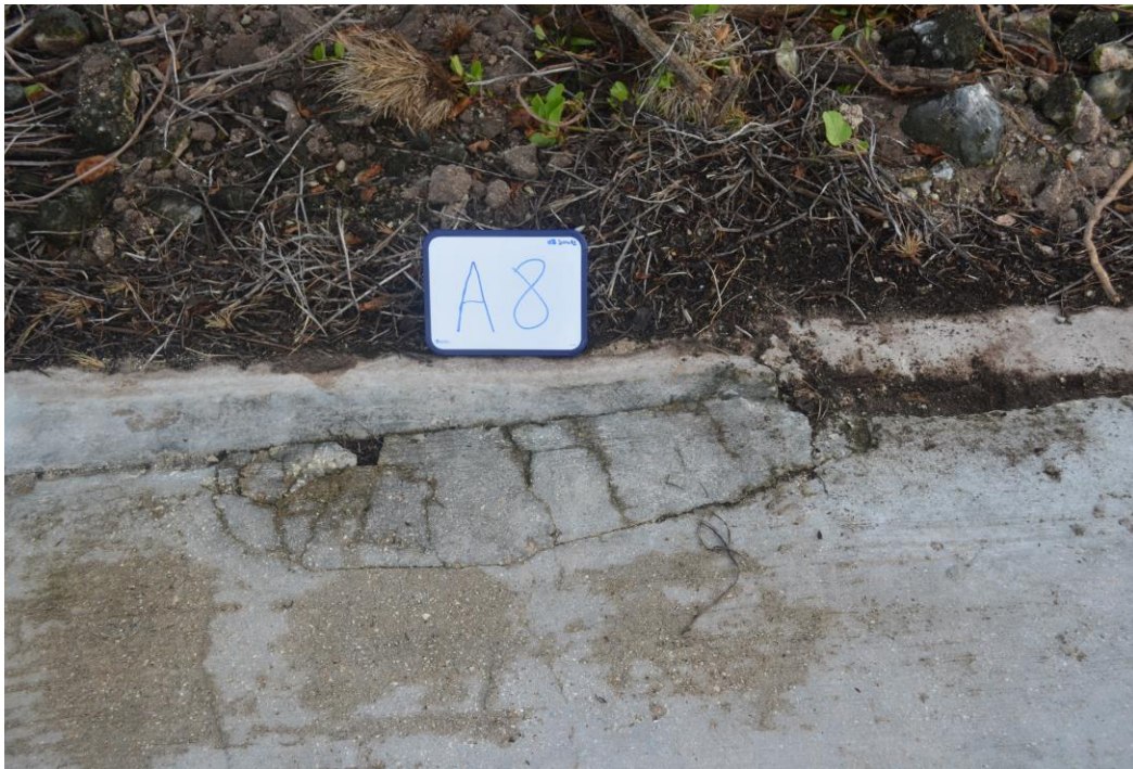
Fig. 21. Cracked concrete with minor spalling along the seam adjoining the keywall on panel A8.
