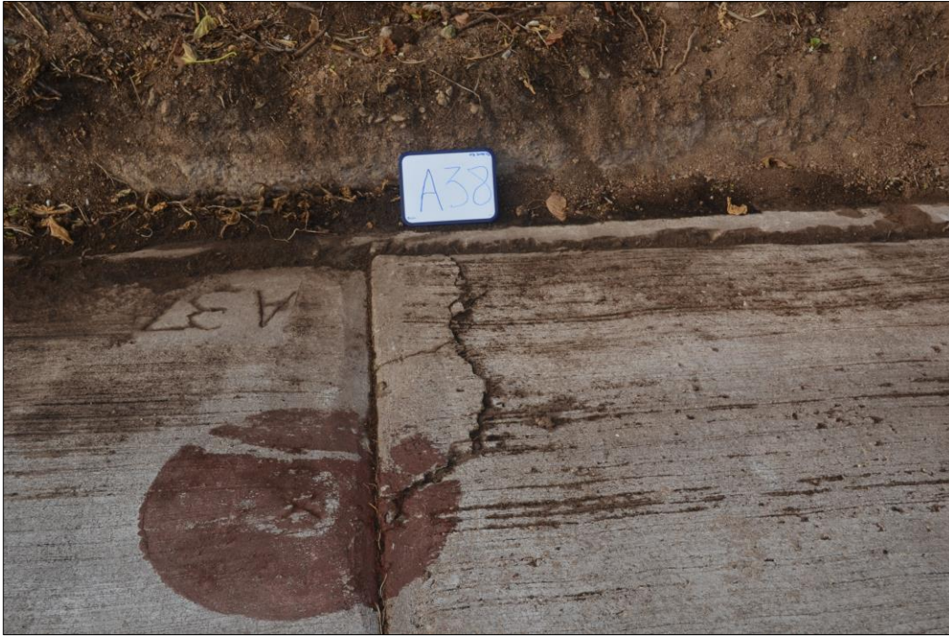
Fig. 28. Cracked concrete with spalled edges on the lower, right-hand corner of panel A38.
