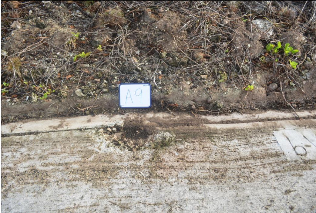
Fig. 22. Spalling of concrete along the seam adjoining the keywall on panel A9.
