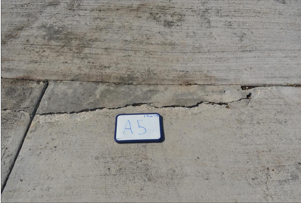
Fig. 20. Cracked concrete with spalled edges on the upper, left-hand corner of panel A5.
