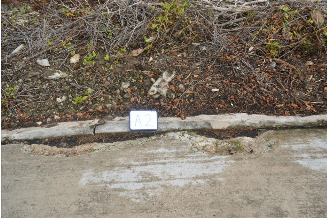
Fig. 18. Spalling of concrete along the bottom seam adjoining the keywall on panel A2.
