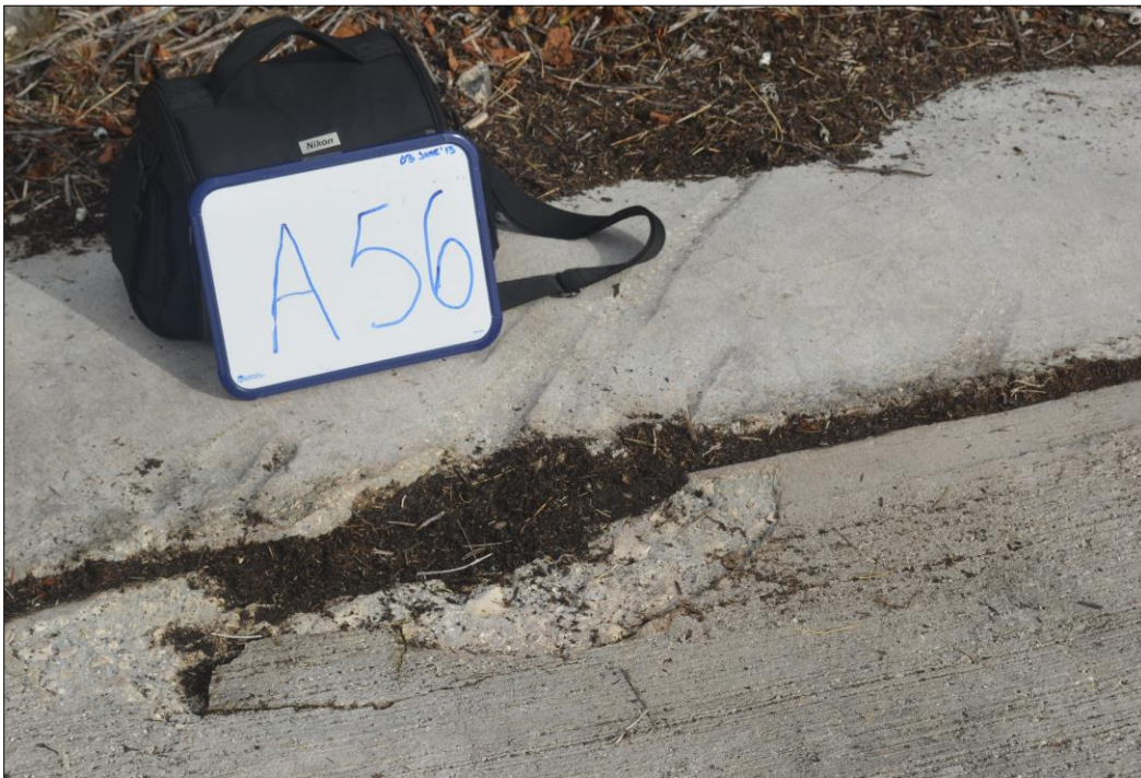
Fig. 31. Spalling of concrete along the seam adjacent to the keywall on panel A56.
