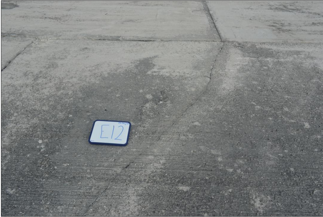
Fig. 39. A visually defective concrete panel (E12) showing a minor to moderate size crack extending upwards across the entire face of the panel segment.
