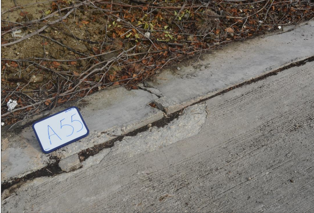
Fig. 30. Spalling of concrete along the seam adjacent to the keywall on panel A55.
