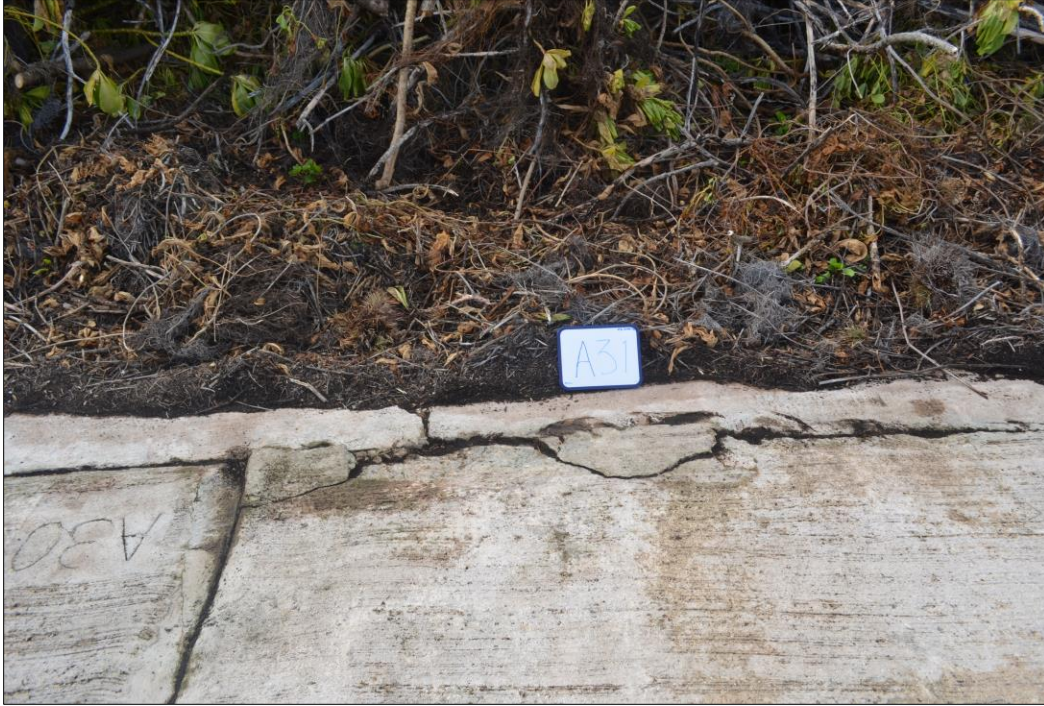
Fig. 26. Spalling and cracked concrete in the bottom right-hand corner and along the seam adjoining the keywall of panel A31.
