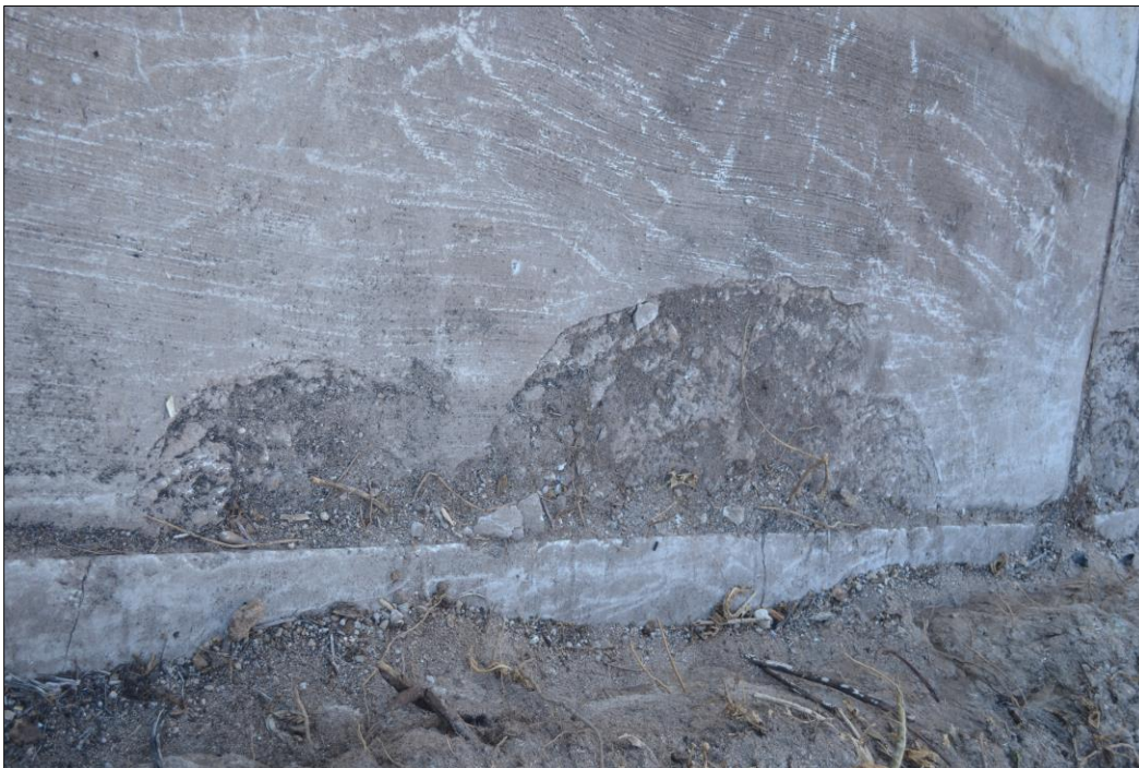
Fig. 25. Spalling of concrete in the bottom right-hand corner along the seam adjoining the keywall on panel A28.
