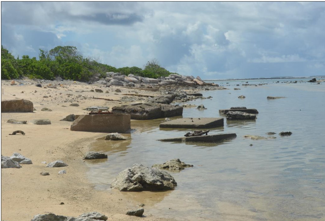
Fig. 4b. View of ripwall 'mole wall' from the ocean reef (concrete blocks in the foreground are unrelated to the riprap wall) [Visual Survey, May 2013].
