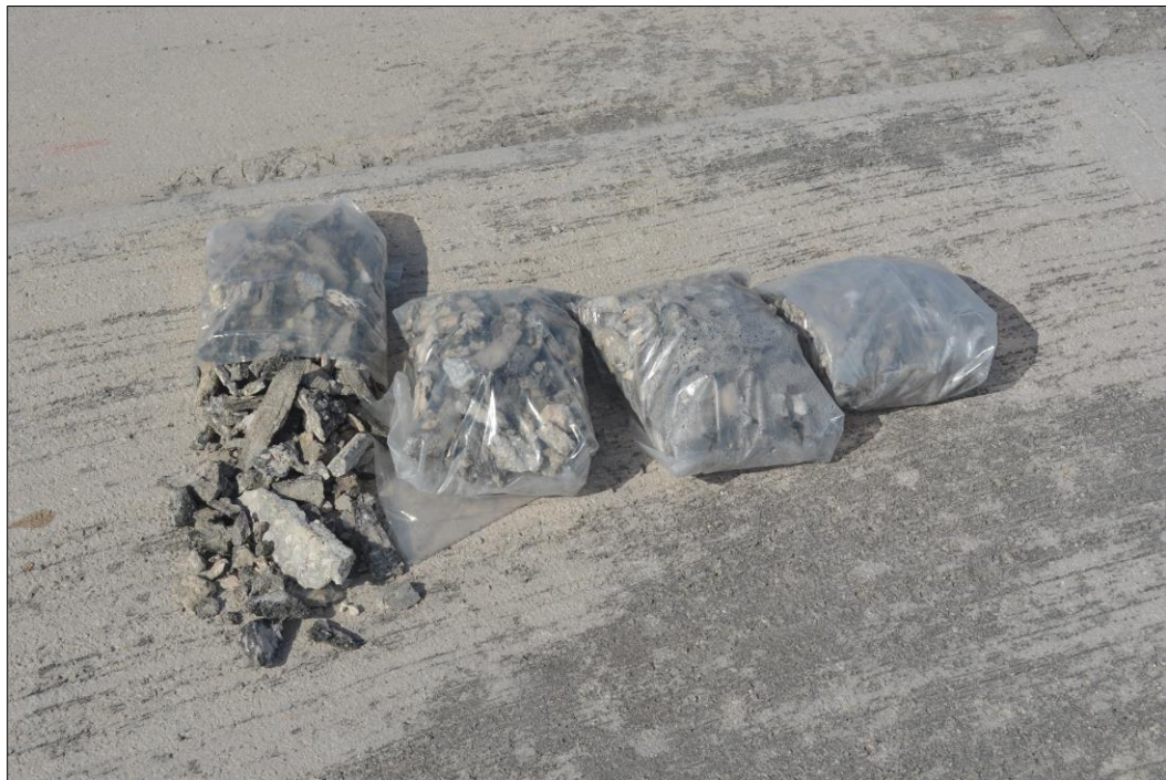
Fig 15. Plastic bags of concrete rubble and other loose debris collected from around Runit Dome (Visual Survey, May 2013) [The volume of debris collected could potentially be used to assess the extent of spalling of concrete between surveys].
