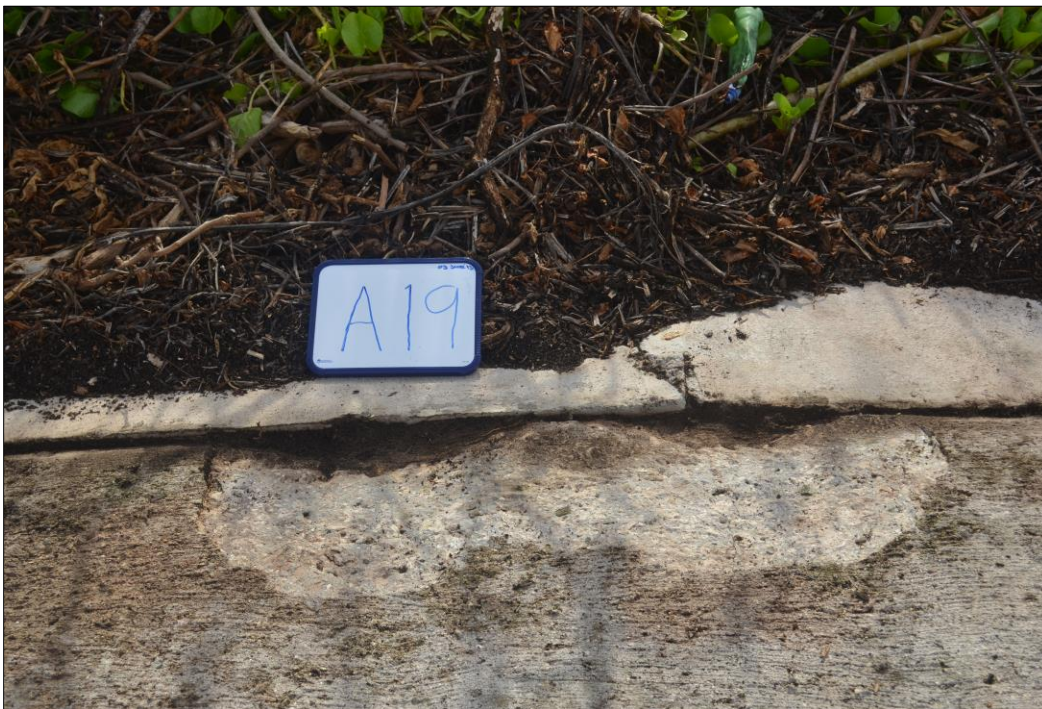
Fig. 23. Spalling of concrete along the seam adjoining the keywall on panel A19.
