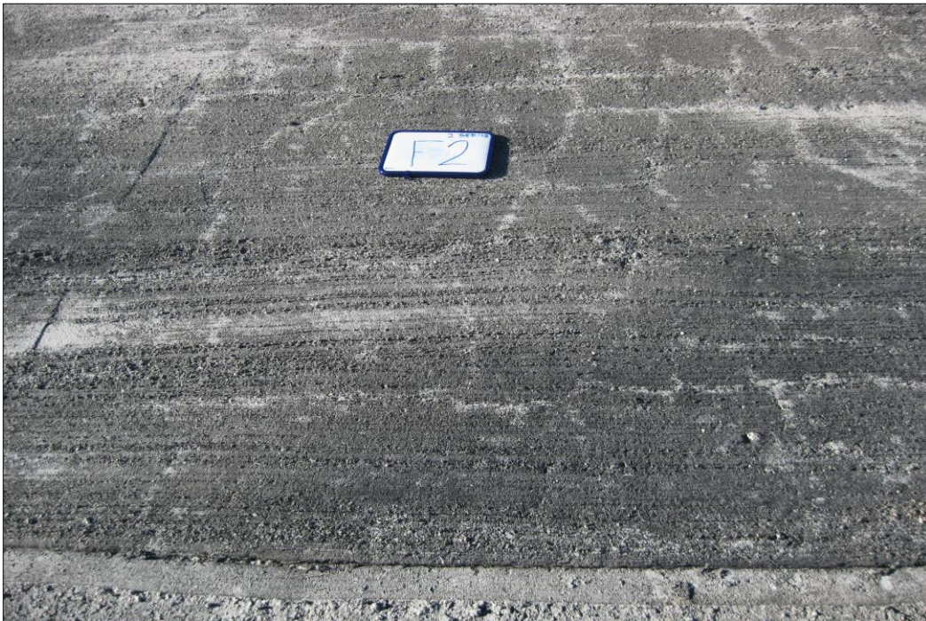
Fig. 37. A visually-defective concrete panel (F2) showing numerous minor surface cracks.
