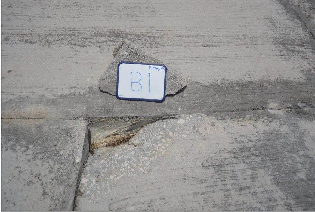
Fig. 32. Major spalling of concrete on the lower, right-hand corner of panel B1.
