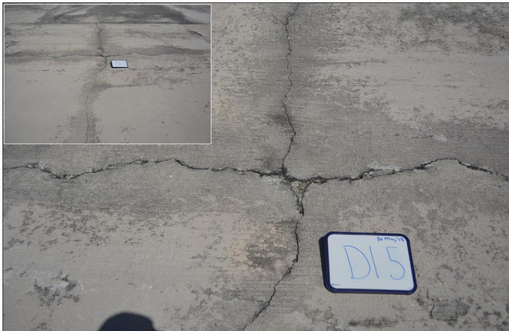
Fig. 40. A more severely cracked concrete panel (D15) with chipped “spalled” edges along the cracks.
