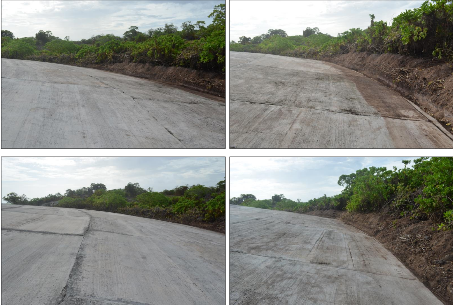
Fig 13. View of Runit Dome after removal of vegetation, dirt and debris (Final conditions, Visual Survey 2013).
