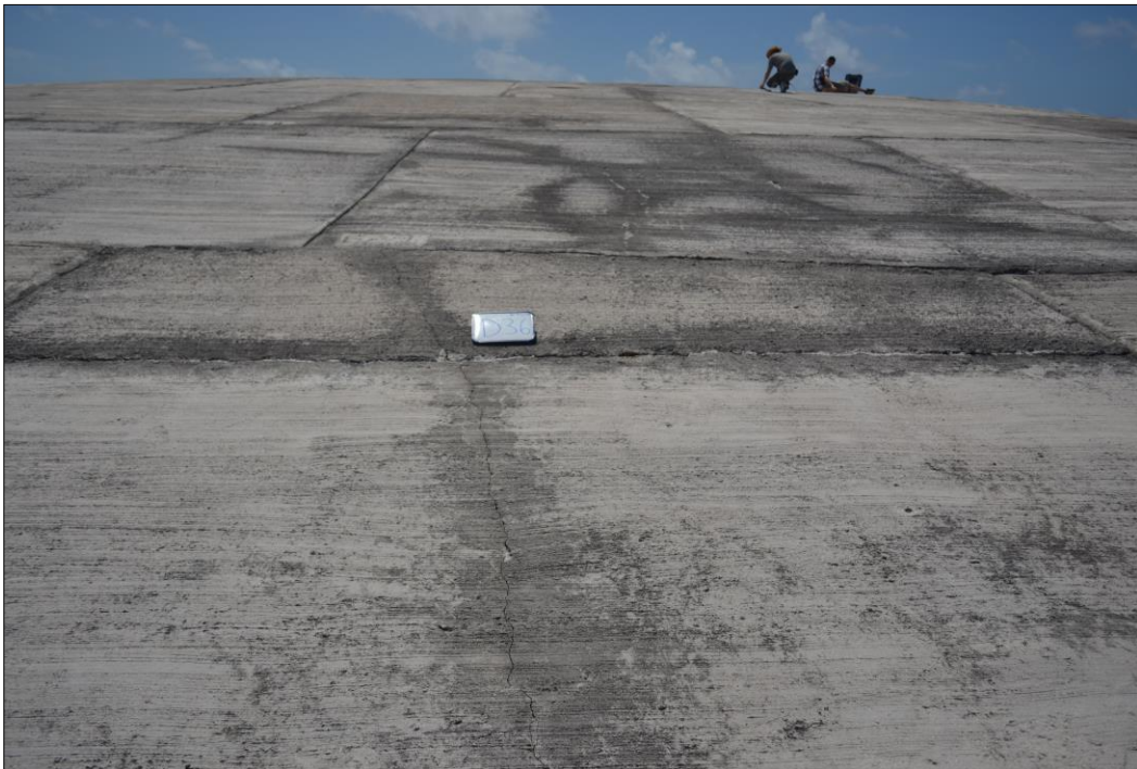
Fig. 17. Concrete panels showing streaks of discoloration running along crack lines.
