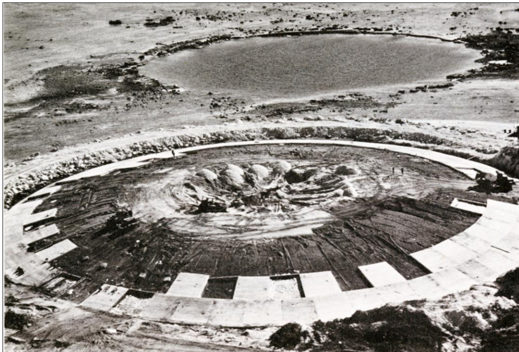
Fig 2. View of the Cactus crater containment structure during construction of individually formed concrete panels [The Lacrosse crater can be seen in the background].
