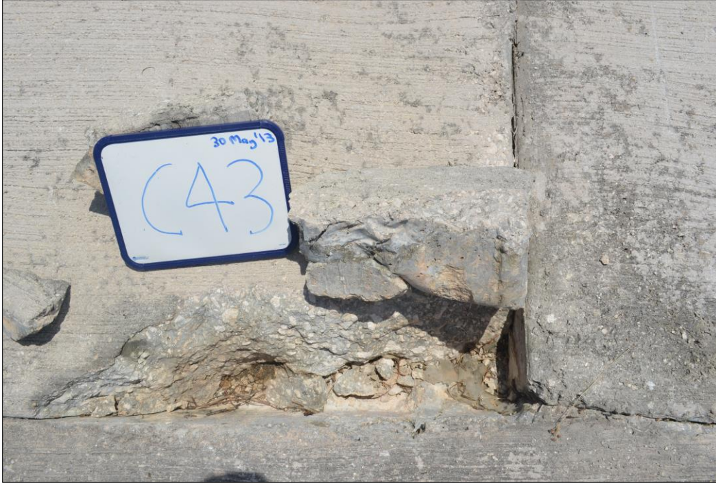
Fig. 36. Major spalling of concrete on the lower, right-hand corner of panel C43.
