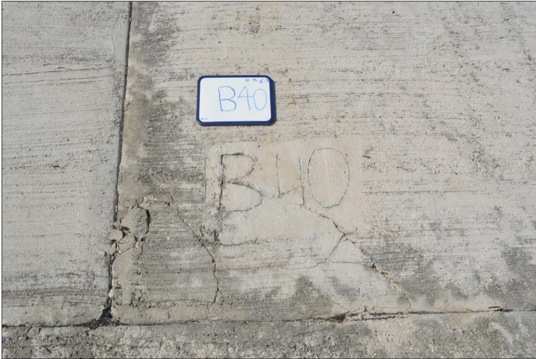
Fig. 33. Cracked concrete with spalled edges on the lower, left-hand corner of panel B40.
