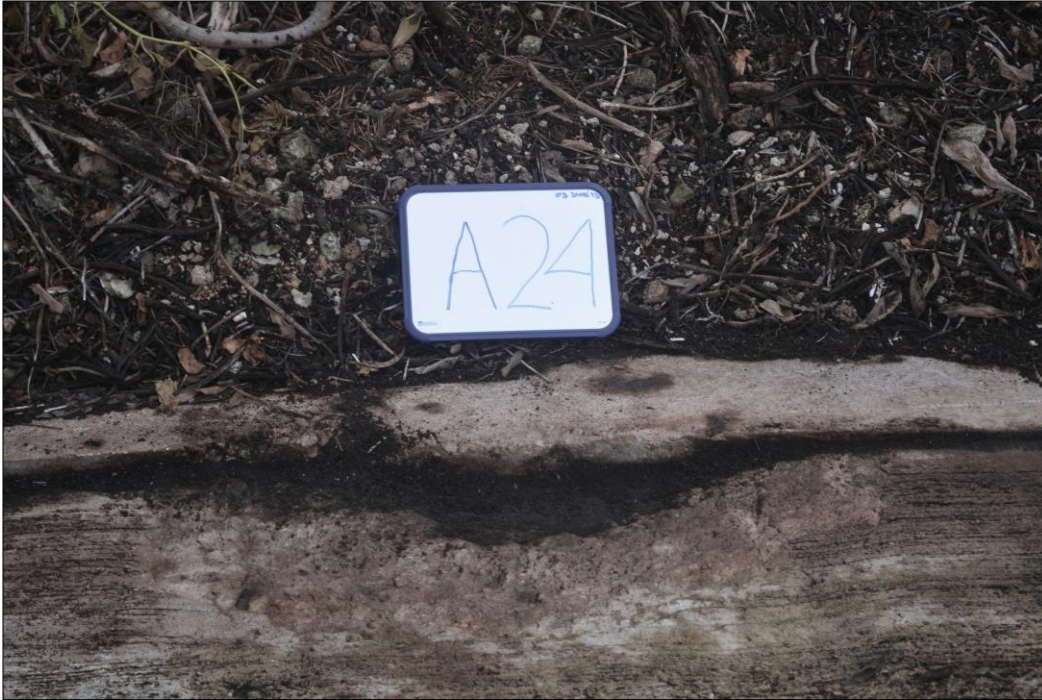
Fig. 24. Spalling of concrete along the seam adjoining the keywall on panel A24.
