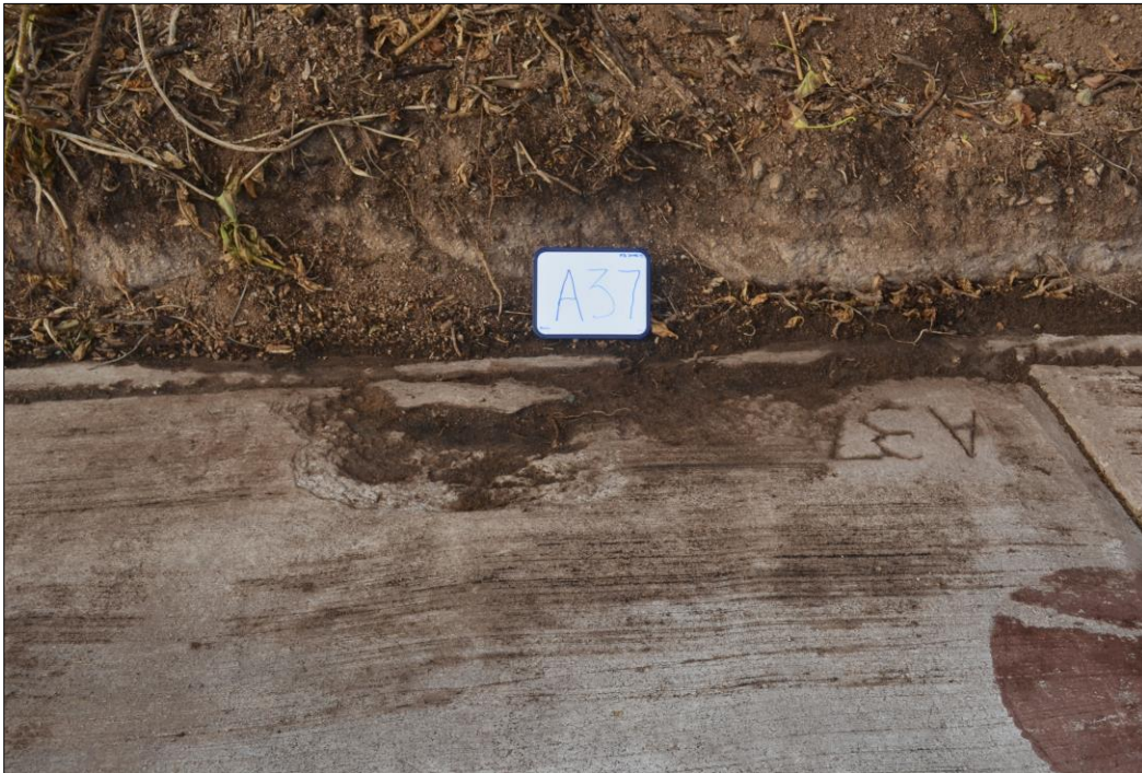
Fig. 27. Spalling of concrete along the seam adjacent to the keywall in the bottom right-hand corner of panel A37.
