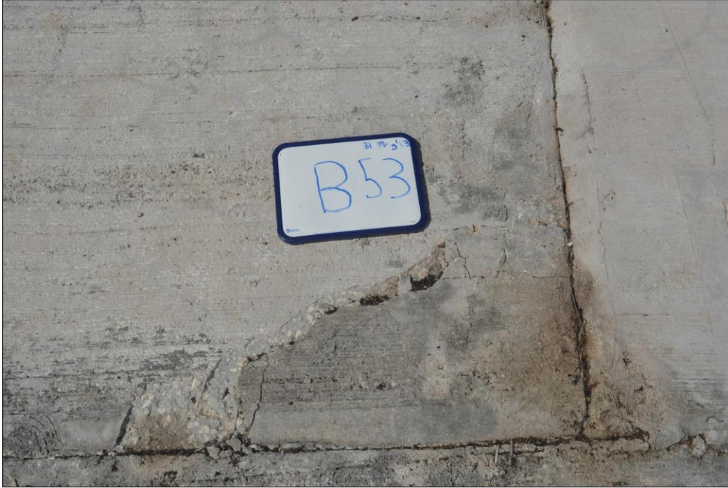
Fig. 34. Cracked concrete with spalled edges on the lower, right-hand corner of panel B53.
