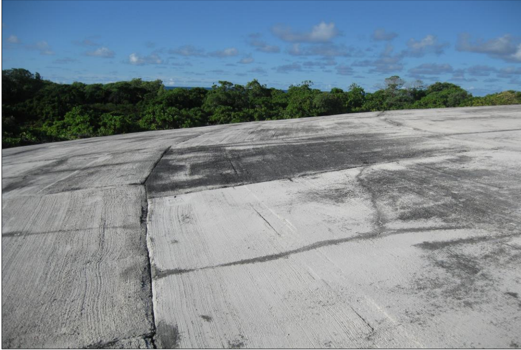
Fig 16. A concrete panel (center) showing signs of weathering and discoloration.
