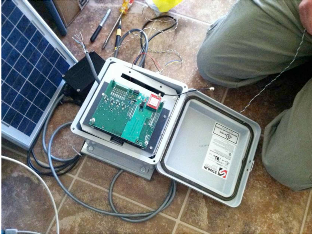
Figure 4. GTMS_V1.0 electronics and enclosure.
