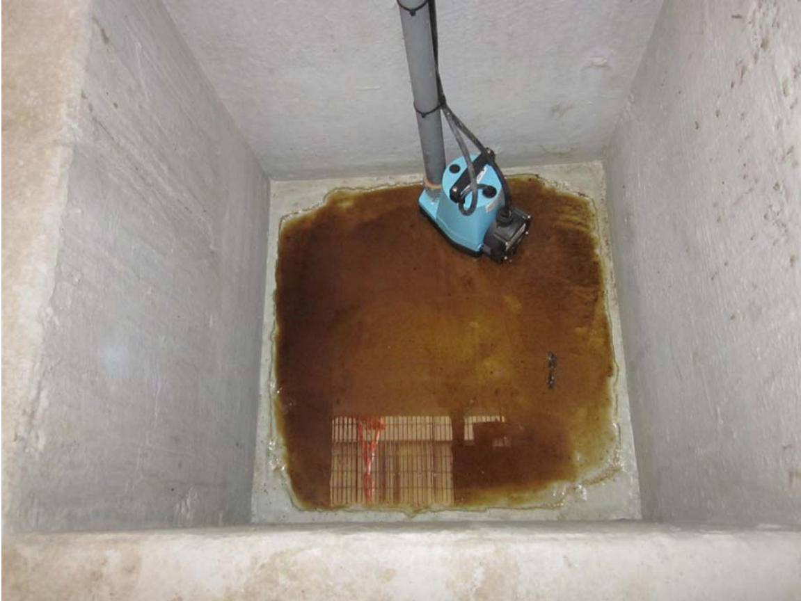
Figure 3. Secondary Containment Sump
