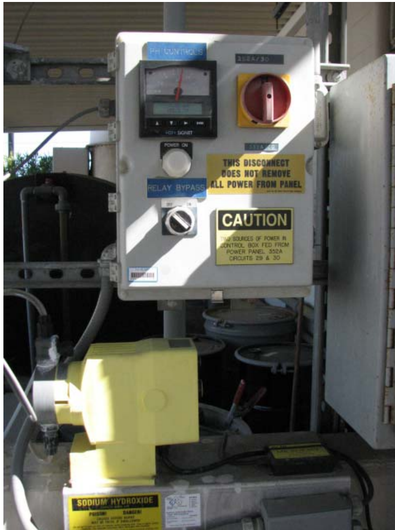
Figure 11. Sodium Hydroxide Injection Pump and Neutralization System Control Panel
