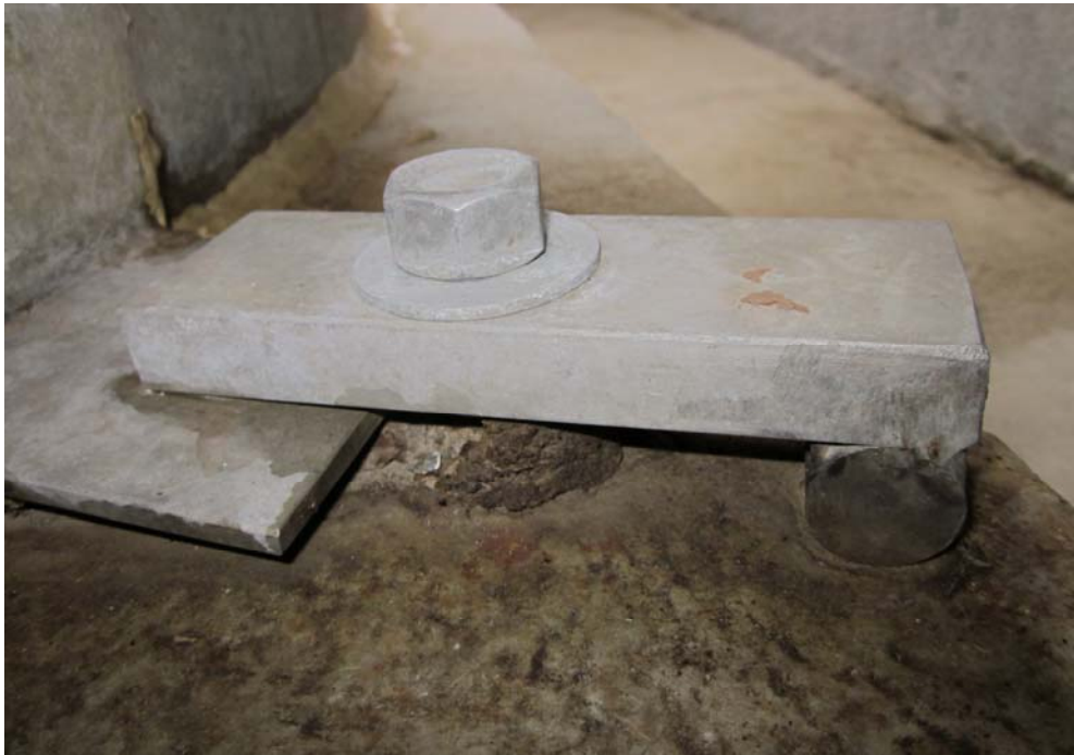
Figure 6. Retention Tank Restraint
