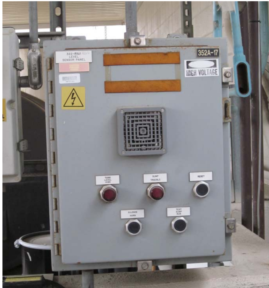
Figure 10. Sump Pump Alarm Panel
