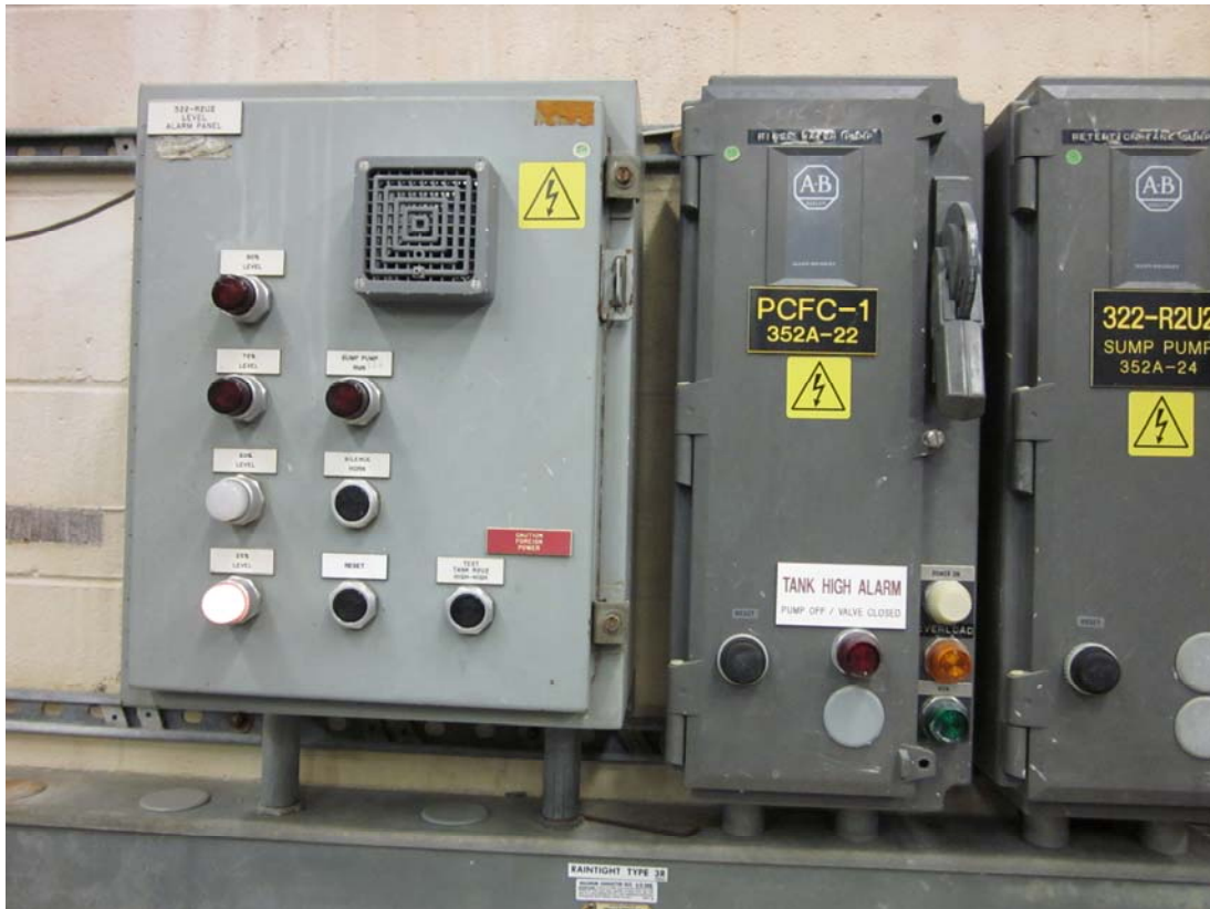
Figure 9. 322-R2U2 Retention Tank Control Panel
