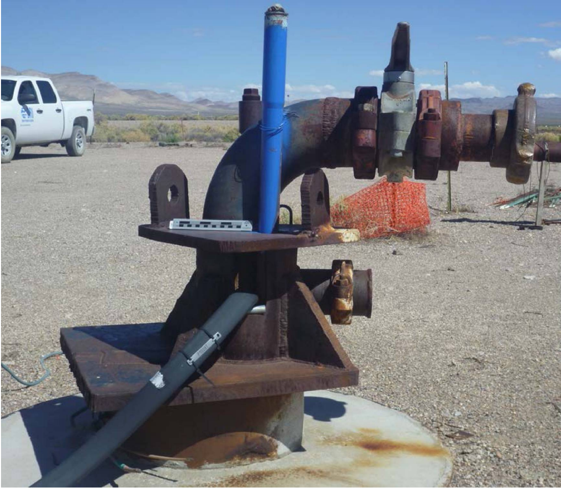
Figure 22. Photo of wellhead configuration for RNM-2s with view looking north.
