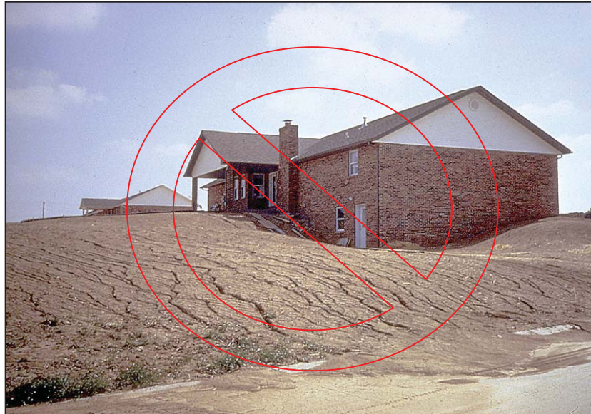
Note that the exposed slope was graded with no tracking. This allowed storm water runoff to concentrate and form rills in the soil.
