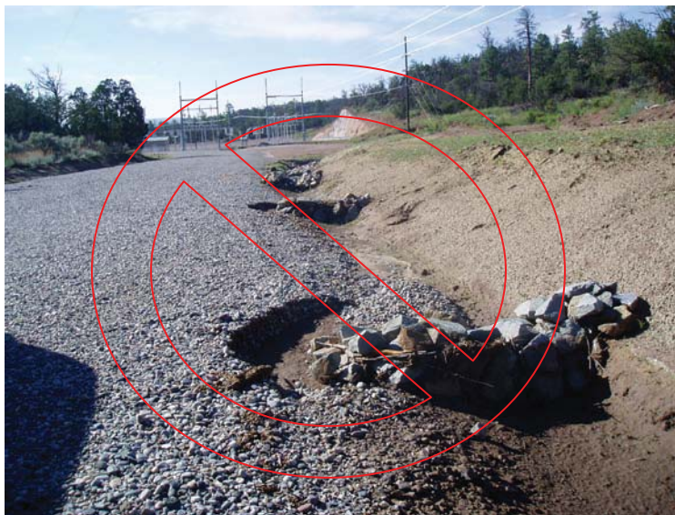
Notice how runoff bypassed the check structures. Channel banks must be sufficient to withstand flows and the dam center must be lower to allow flow over the check dam.
