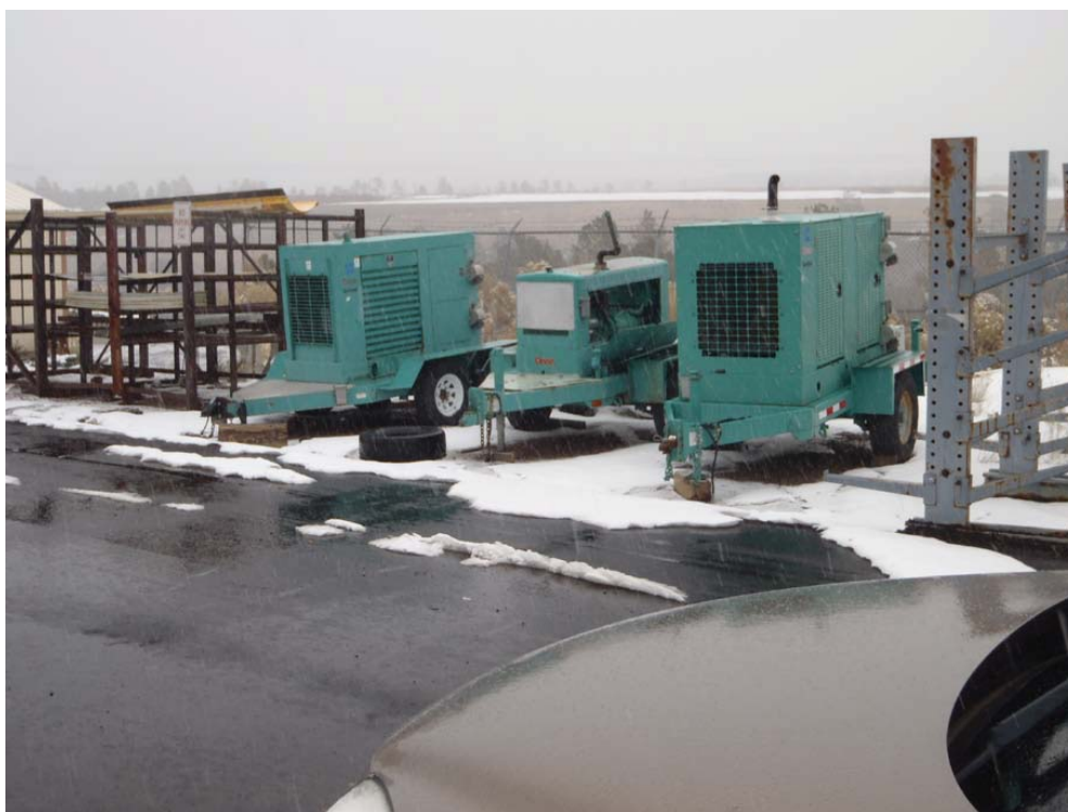
Stored equipment can leak fluids
