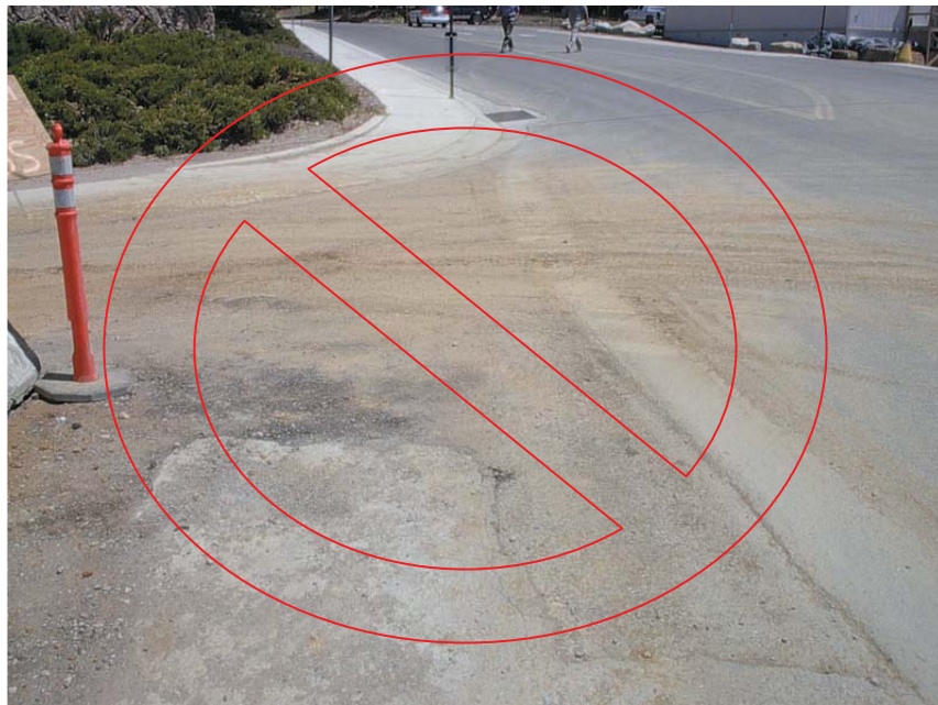
Failure to install a construction entrance has lead to sediment transport offsite.
