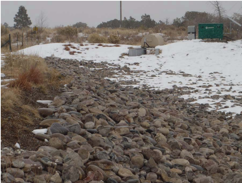
Rock and filter fabric lined detention pond to collect storm water
