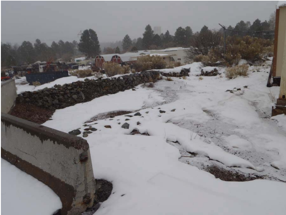
Berm channeling storm water flow
