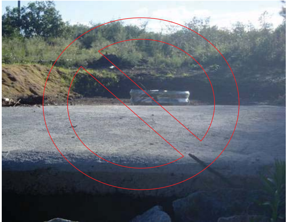
Standpipe overflow height is higher in elevation than the basin spillway.
