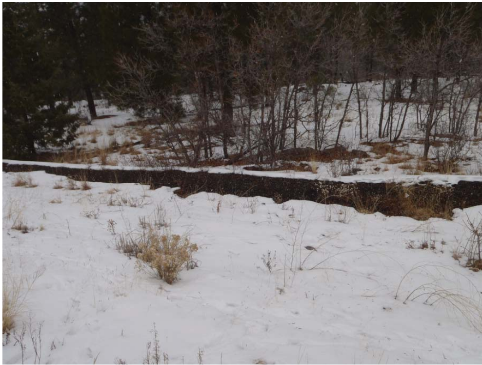
An asphalt berm (north of Roads and Grounds west) to channel storm water and prevent sediment transport
