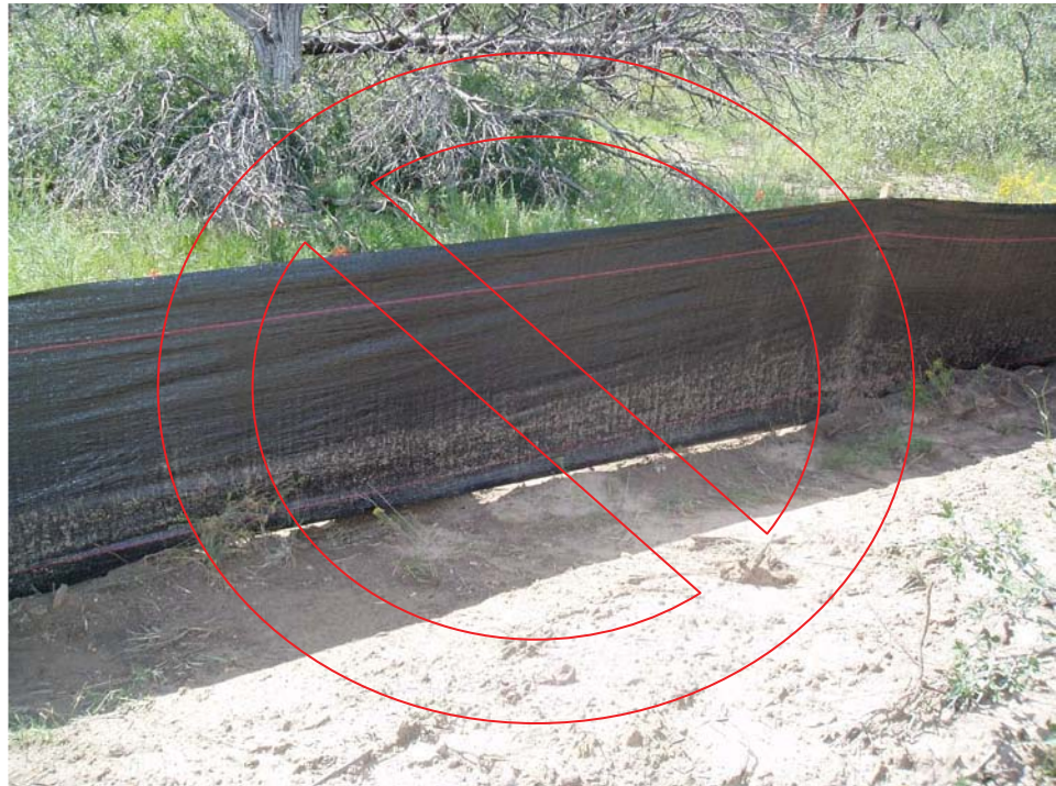
Silt fence should be properly entrenched for proper operation.
