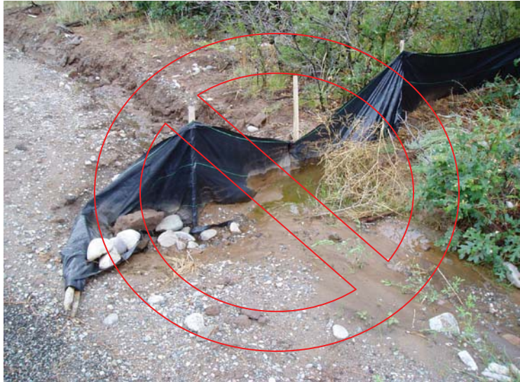
Silt fence cannot be used as a check structure and is not designed for concentrated flow.
