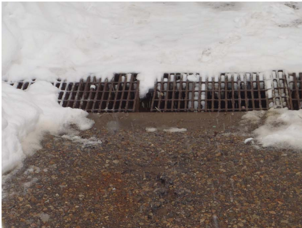
Trench drain that transports storm water UNCLASSIFIED
