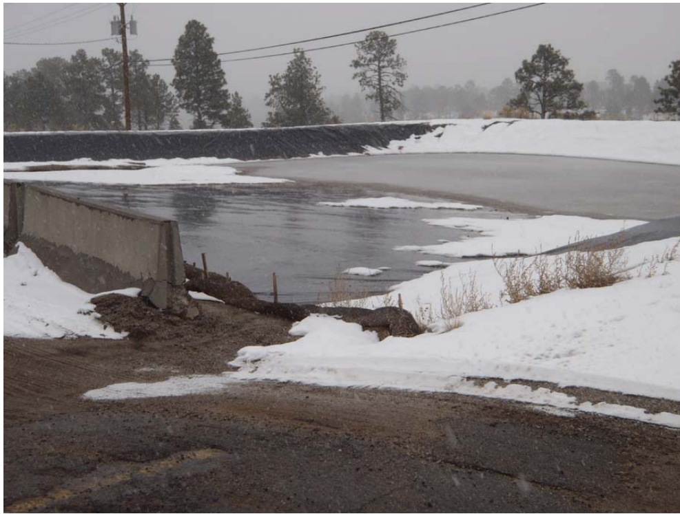
This lined pond was constructed to contain the release of salt from the salt shed
