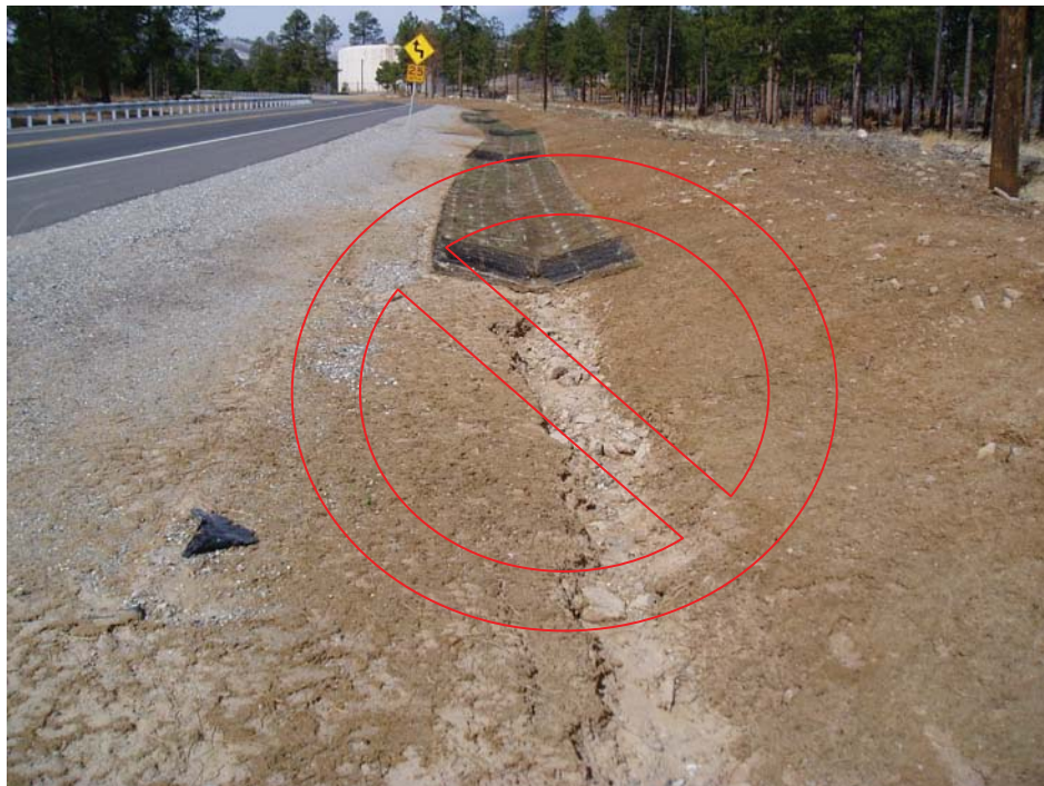
TRM installation was not continued along swale where water flow is concentrated, causing erosion.
