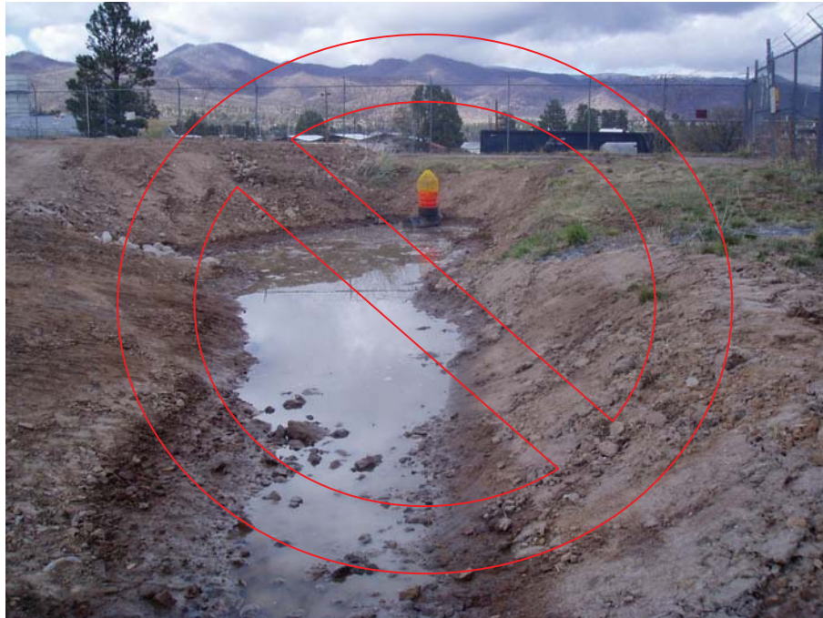
Embankments of pond should be stabilized following initial grading of pond.
