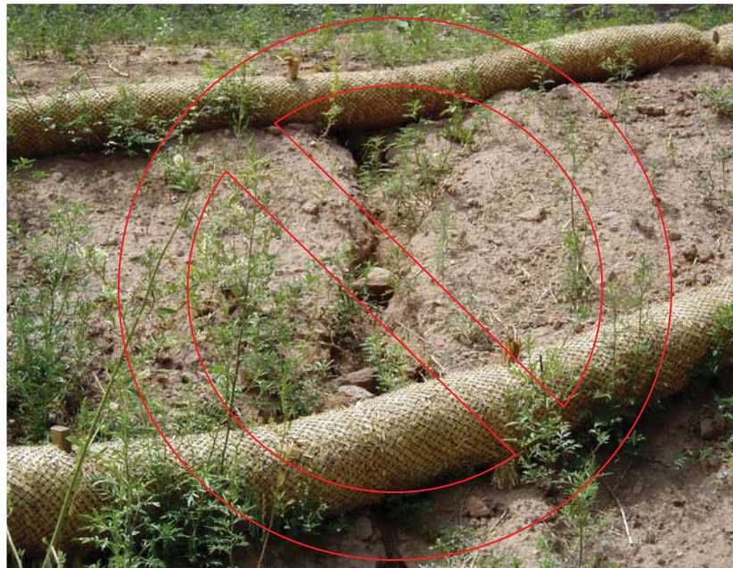
A rill is forming under the fiber roll. The rill should be filled in. The fiber roll should be properly entrenched into the soil so that water velocity is decreased and water is forced to pool behind to promote sedimentation and flow over the fiber roll.
