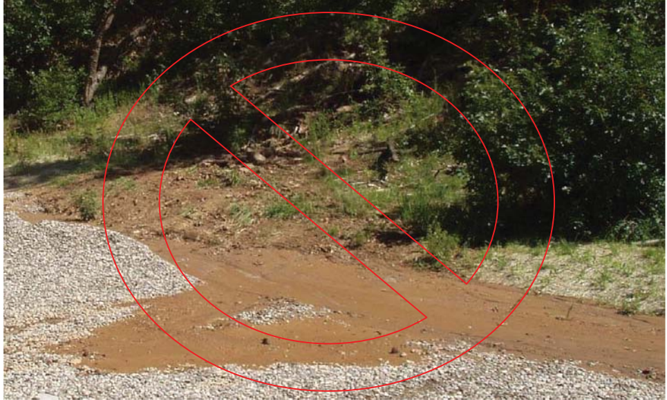
Berm was not well stabilized and could not stand up to run-on flows. Berms and swales should be designed and constructed to handle site specific run-on or run-off flows.
