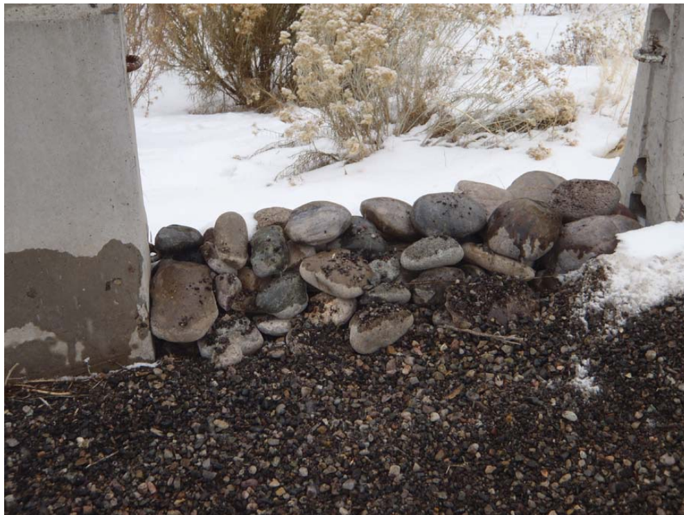
Rock check dam between two Jersey barriers to slow storm water velocity and prevent sediment transport
