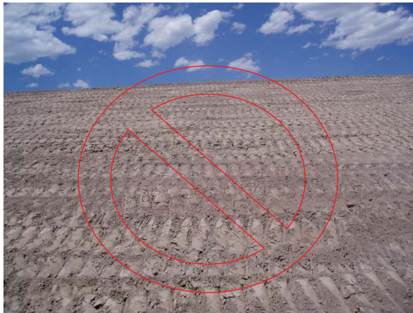
Note that the slope was track-walked in the wrong direction. This will cause rills to form as water will be allowed to follow the grooves in the soil and gain velocity causing erosion. Track walking with machinery up and down the slope creates grooves that will catch seed and fertilizer and will promote mulch cover to stay on the slope. It will also slow water velocity and reduce runoff and erosion.
