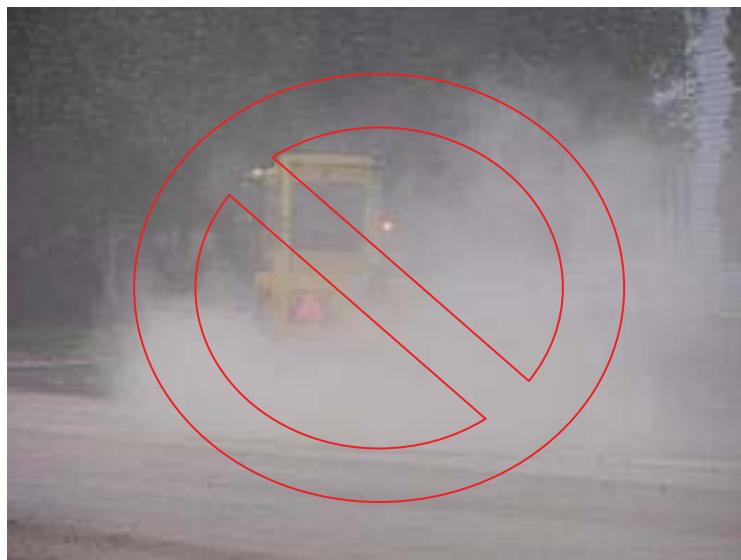
Dust control was not applied sufficiently.
