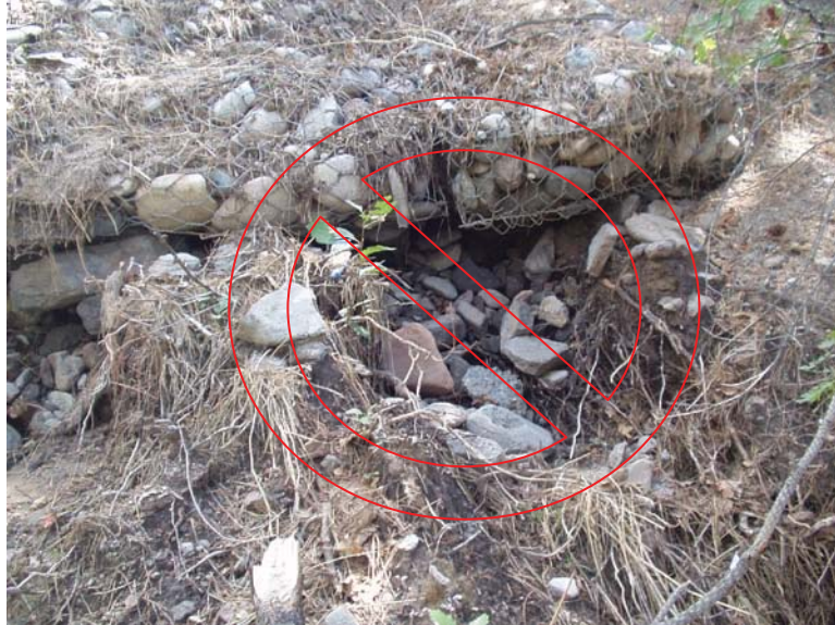
Obstructions not removed from channel before gabion was installed. No filter fabric under the gabions. Scour under the gabions.
