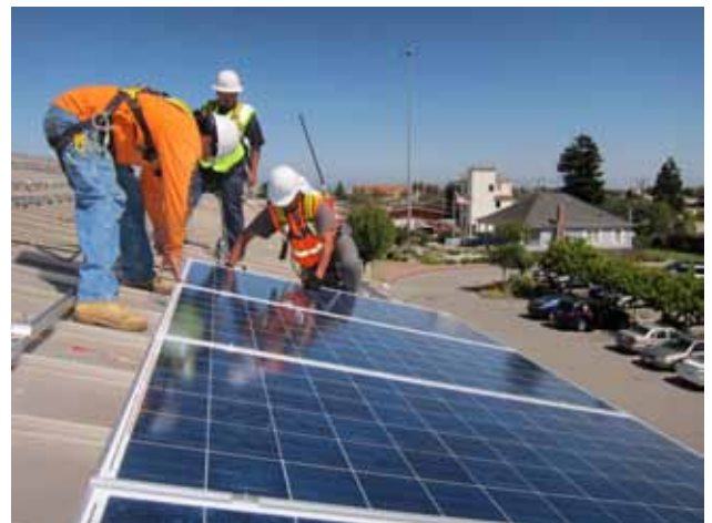
Millbrae Library Solar Panels. Siemens Building Industries and Luminalt Solar Energy Solutions. Kent Fields Photography.
