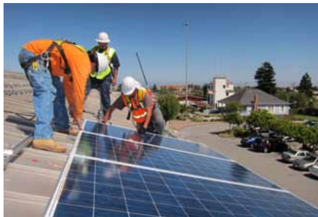
Millbrae Library Solar Panel Installation, Siemens Building Industries, Luminalt Solar Energy Solutions. Kent Fields Photography.
