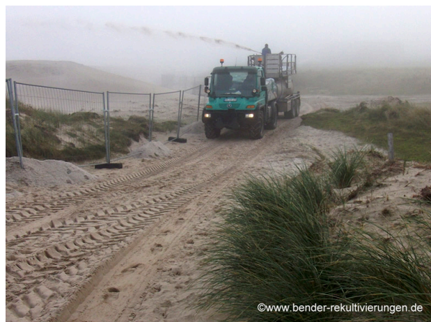
Surface stabilization for dust control at an industrial site using soil binding agents applied by a hydroseeder. Source: Bender GmbH & Co.KG.
