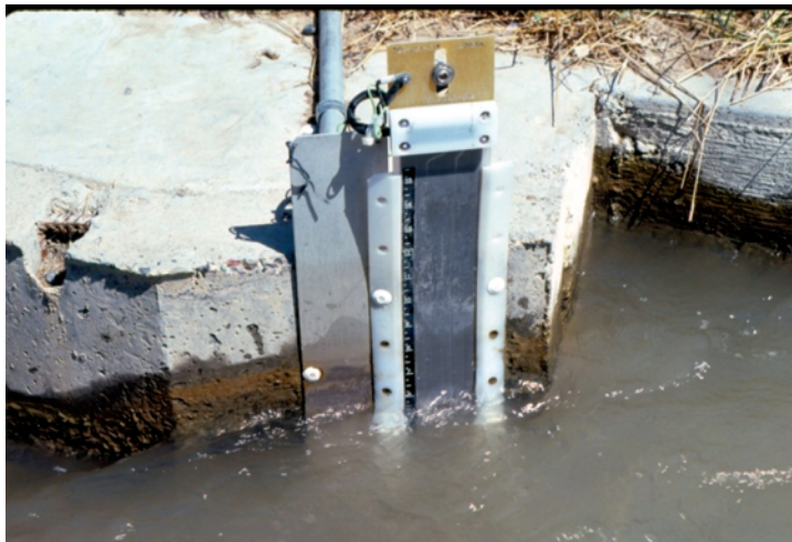
Figure 2. Photograph of a linear strip gage installed in an existing concrete weir.
