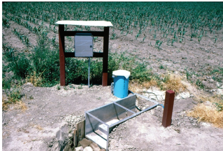
Figure 4. Photograph of a typical inflow installation with a stilling well and float potentiometer.
