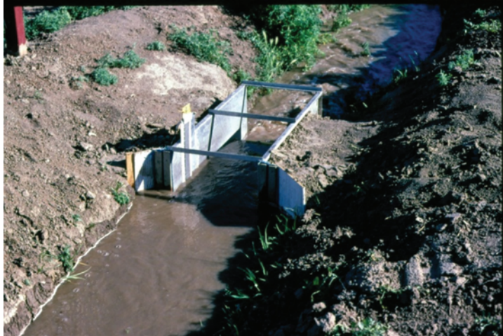
Figure 3. Photograph of a typical installed broad-crested weir with a linear strip gage.
