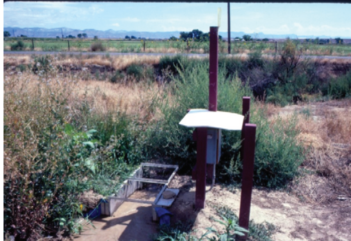
Figure 6. Photograph of a typical outflow installation with pressure transducer.
