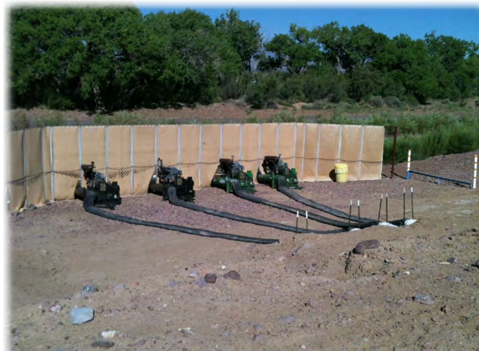
Pumps transferring water from the conveyance channel to the main channel of the Rio Grande near San Pedro; the photograph was taken outside the mapped area shown. Photograph by Daniel K. Pearson, U.S. Geological Survey, June 9, 2012.
