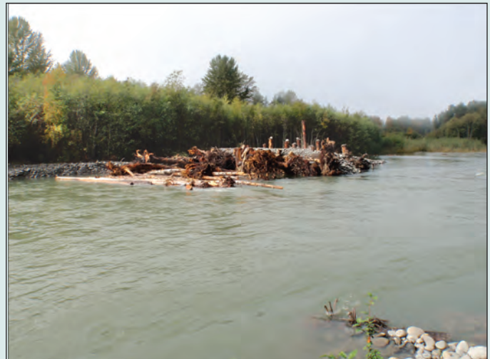
Figure S3.1.1. Newly constructed engineered log jam on the Elwha River, Washington during winter flooding 2009. This structure is one of 50 that the Lower Elwha Klallam Tribe has installed in the lower Elwha River prior to dam removal.
