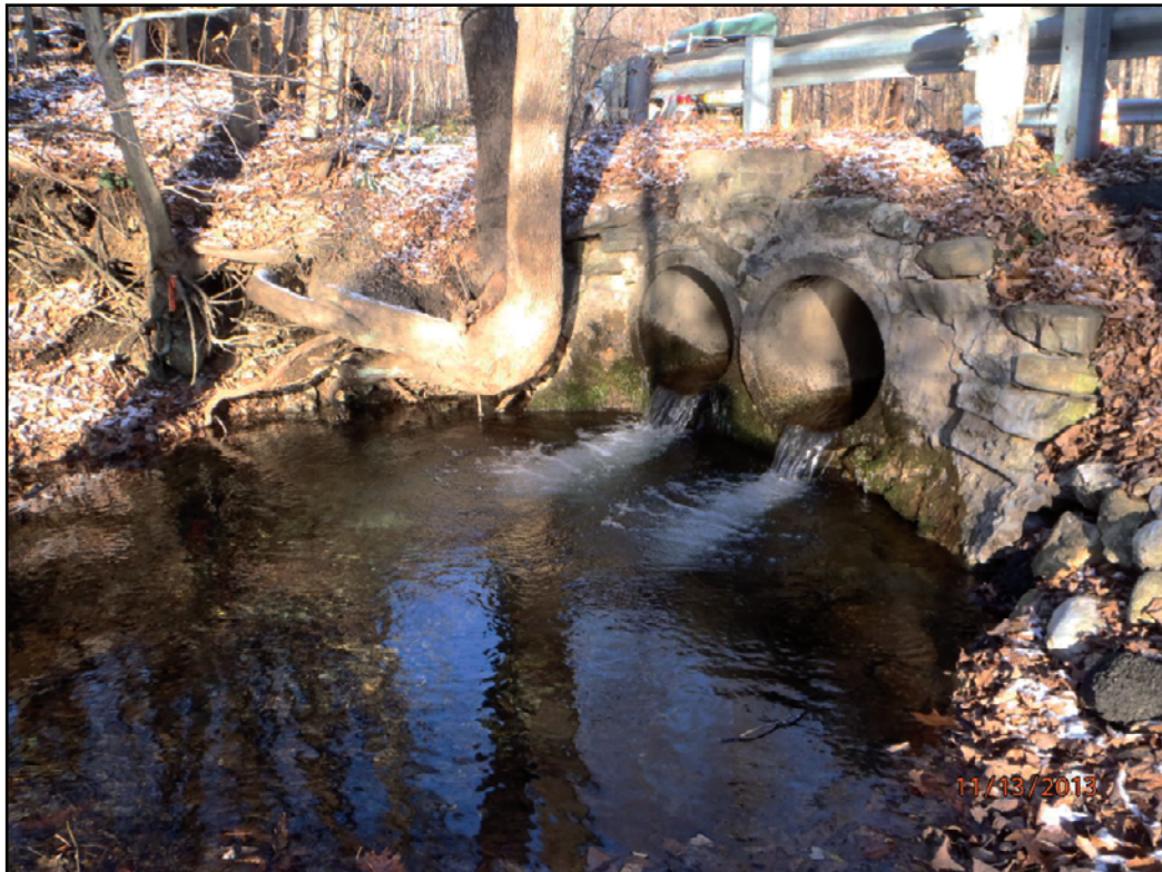
Figure 7. Downstream faces of Churchill Brook crossings in Pittsfield, Massachusetts at A, Churchill Street, and B, Hancock Road.
