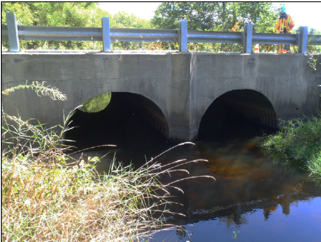
Figure 3. Upstream face of Main Street (Route 27) crossing Nashoba Brook in Acton, Massachusetts.
