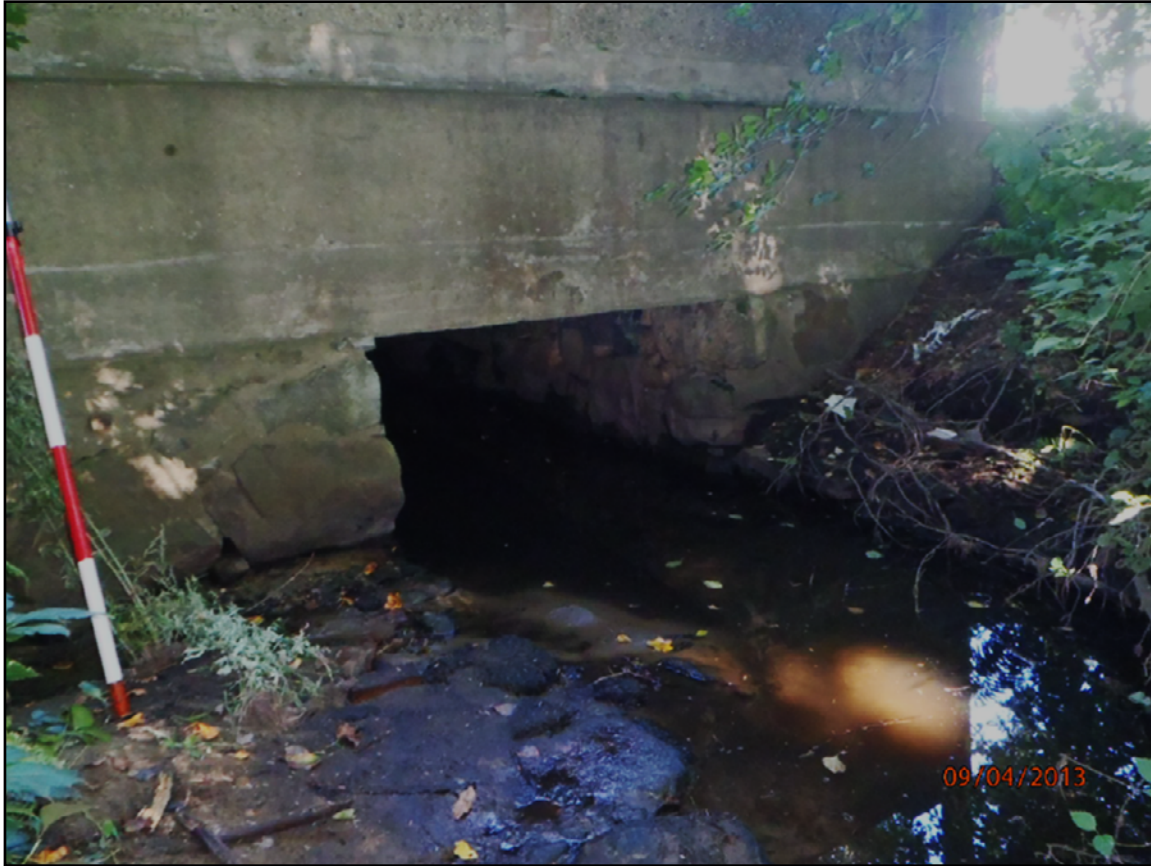
Figure 2. Downstream face of Church Street (Route 62) crossing Mill Brook in Wilmington, Massachusetts.
