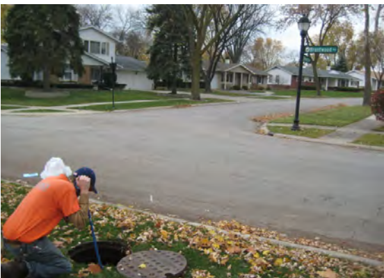
Figure 5. Photographs showing sanitary sewer line inspection and upgrade operations in the study area, Elk Grove Village, Illinois. A , Camera inspection of the trunk line near observation well TW7. B , Cured-in-place lining operation of the trunk line near well TW7. C , Study-related inspection of a manhole near well TW9 by U.S. Geological Survey staff.
