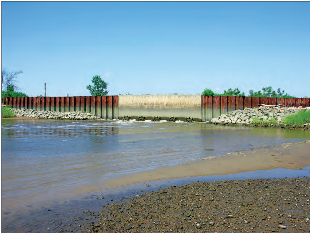
Figure 5. Red Lion Creek tide control structure with reinforced dike and five outflow gates, looking from the Delaware River at low tide in 2010. [Photograph by Todd Keyser, Delaware Department of Natural Resources and Environmental Control.]
