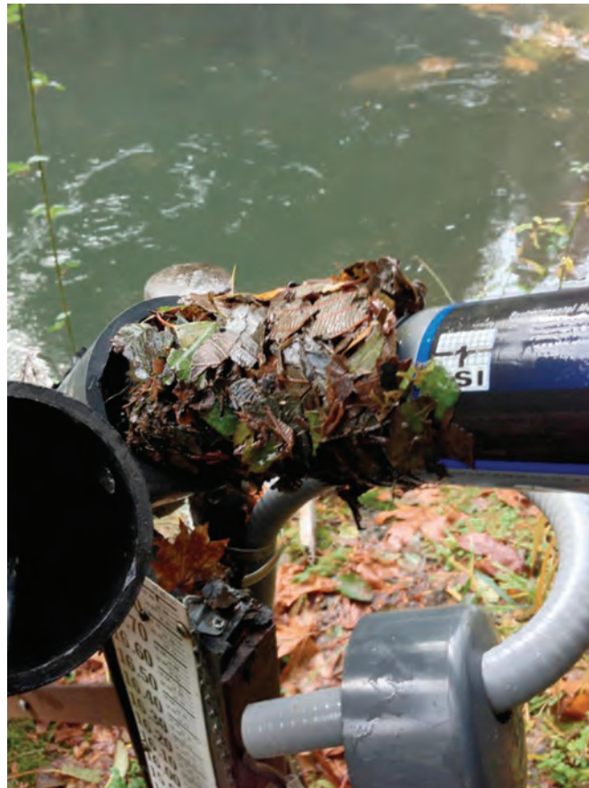
Figure C1. Siltation and leaf compaction clogging the pipe and instrumentation at the Trask River site, northwestern Oregon. Photograph by Mark Uhrich, U.S. Geological Survey, November 2012.
