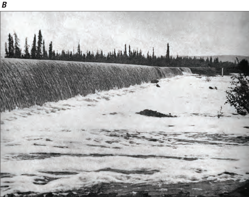
Figure 13. (A) Flood frequency curves and (B) Little Chena River overtopping Bridge 270 at Chena Hot Springs Road, Alaska, during the 1967 flood. Photograph by Fairbanks News-Miner (Childers, 1972).
