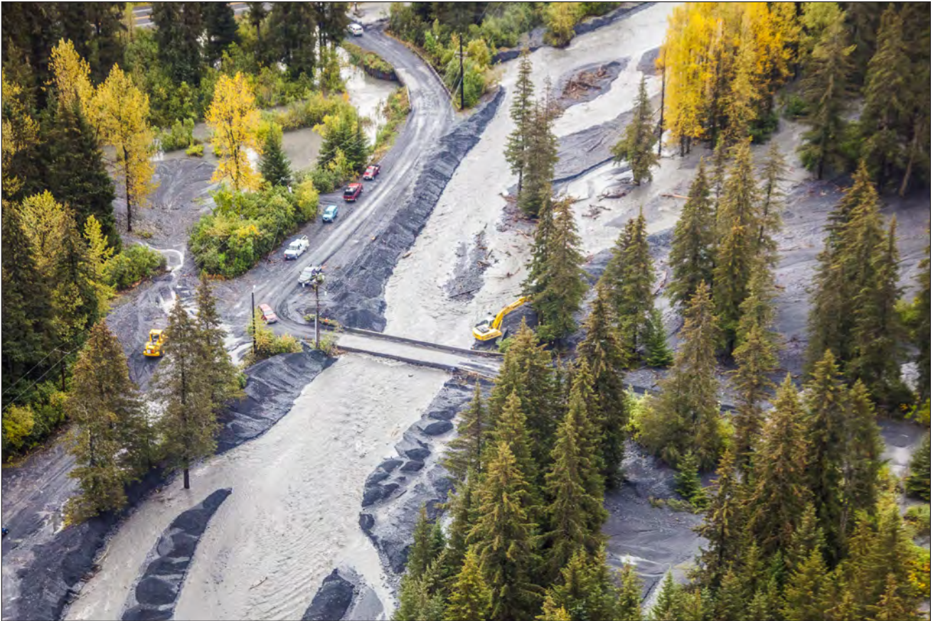
Figure 17. Pressure-flow conditions, dredged channel, and gravel berms at Lost Creek Bridge 1838, near Seward, Alaska, September 21, 2012. Photograph by City of Seward.
