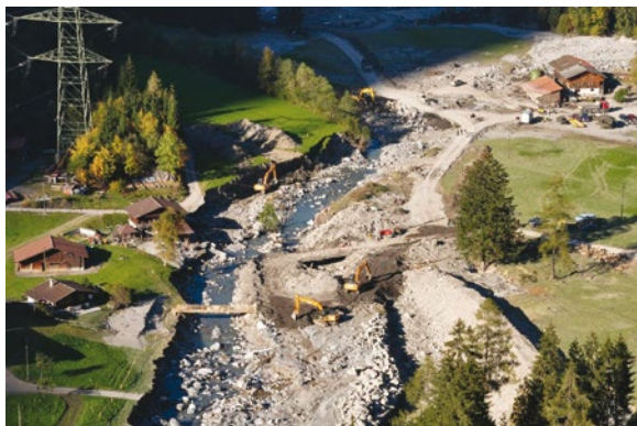
Damage caused by side erosion of the Kander River, Berne, Switzerland, 10 October 2011, Photographer: Hugo Raetzo, Federal Office for the Environment, Switzerland
