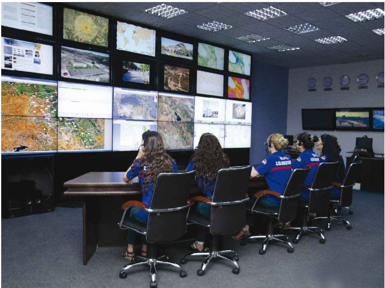
Photograph: Crisis Management Centre and "911" Rapid Response of Armenia's Ministry of Emergency Situations Source: Ministry of Emergency Situations, Armenia
