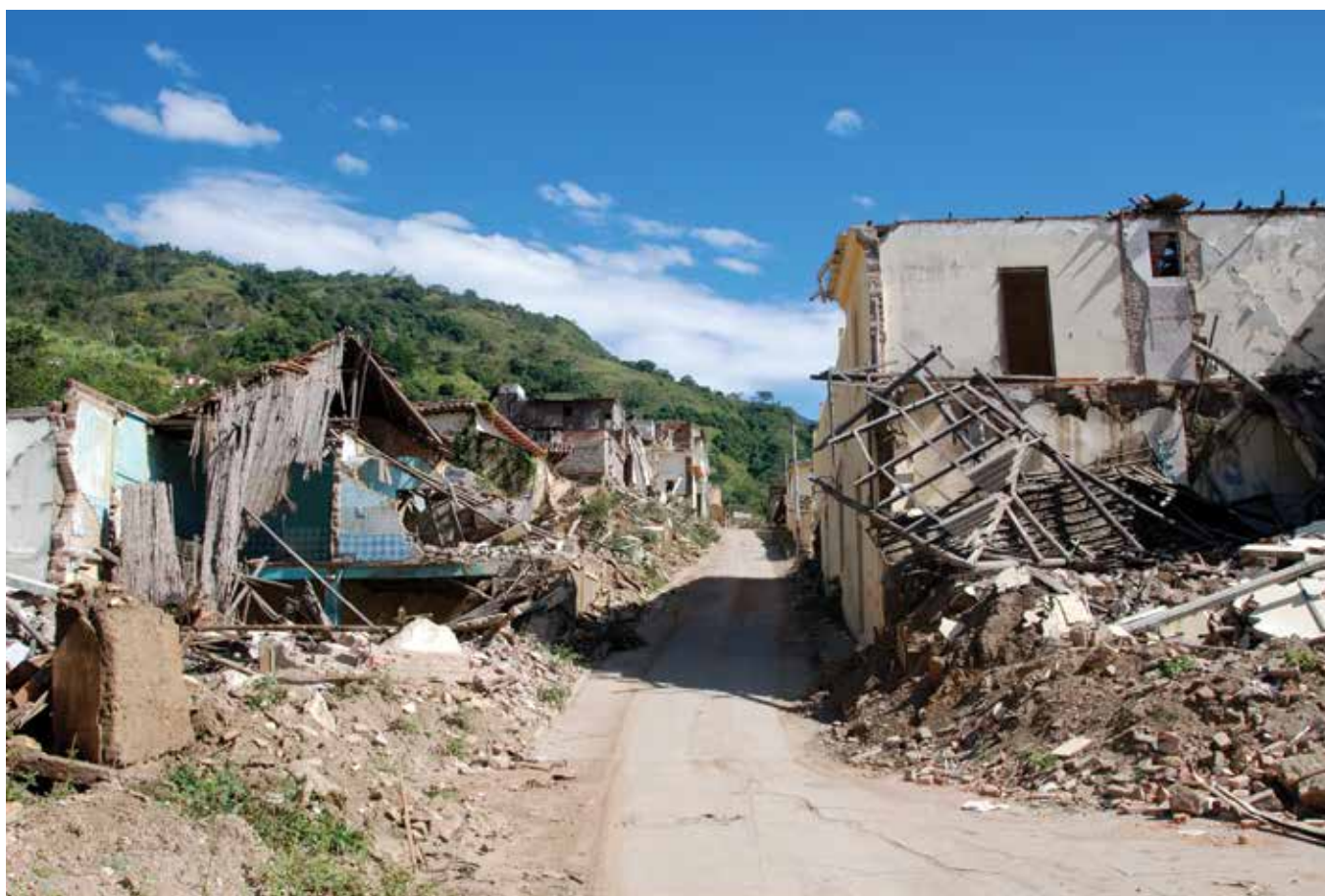
Housing destroyed by landslides. Municipality of Gramalote (Norte de Santander – Colombia), 2011. Photography: Gabriel Jaime Arango Zapata.
